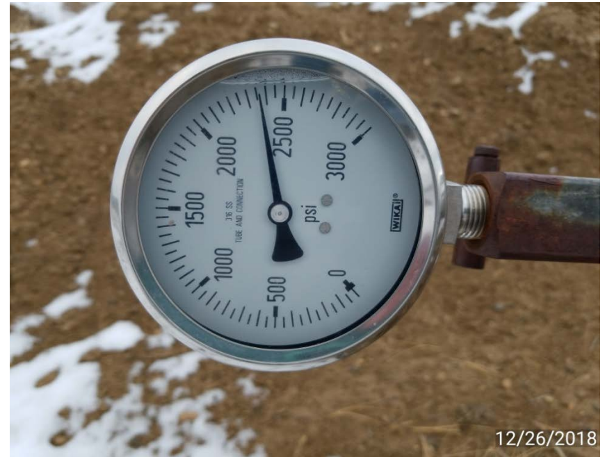
Photo 4. Casing pressure gage on 12-26-2018,
