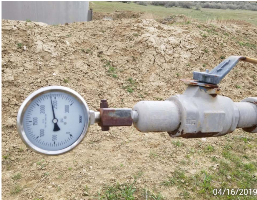
Photo 3. Casing pressure gage on 4-16-2019.
