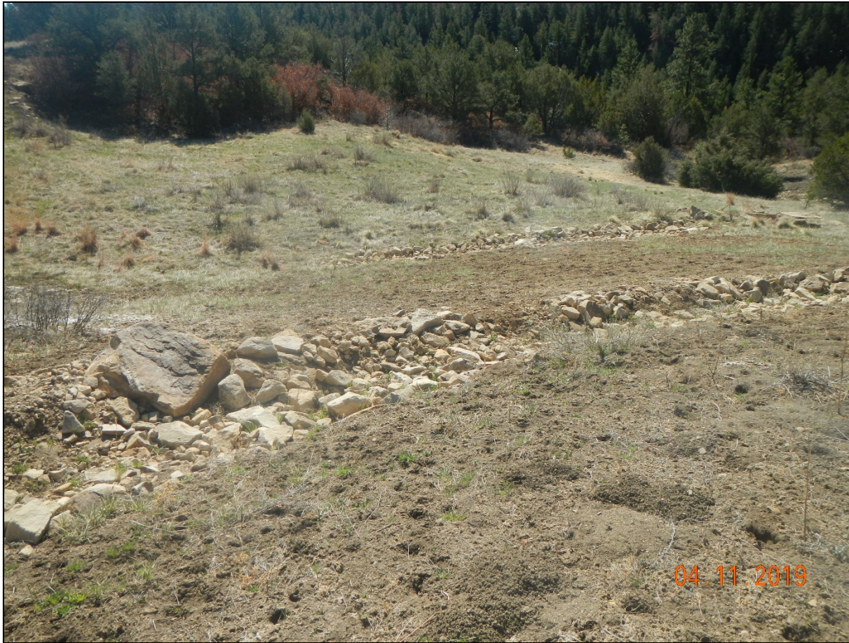
Photo 1. Facing toward the location. Rock rip/rap has been placed diversion ditches. Slope has been reseeded.
