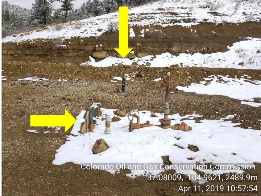
Photo 3 Unused, unmarked and not LOTO risers.
