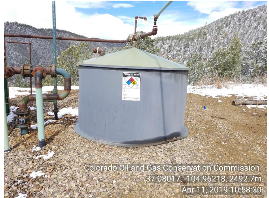
Photo 4 Tank not painted appropriate color
