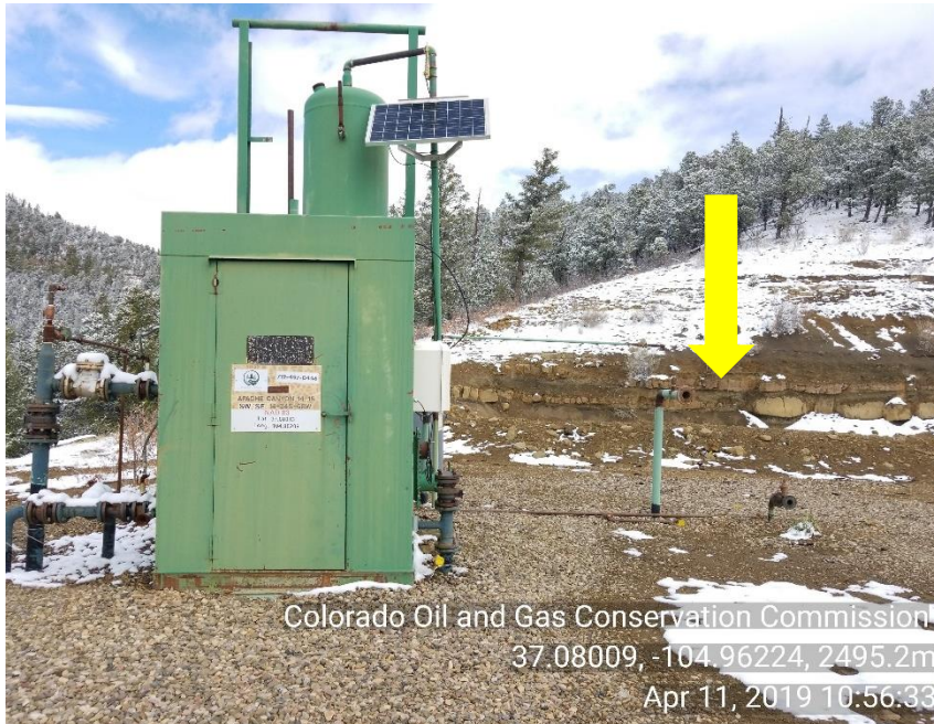
Photo 1 Sep/meter house. Unused, unmarked and not LOTO risers.
