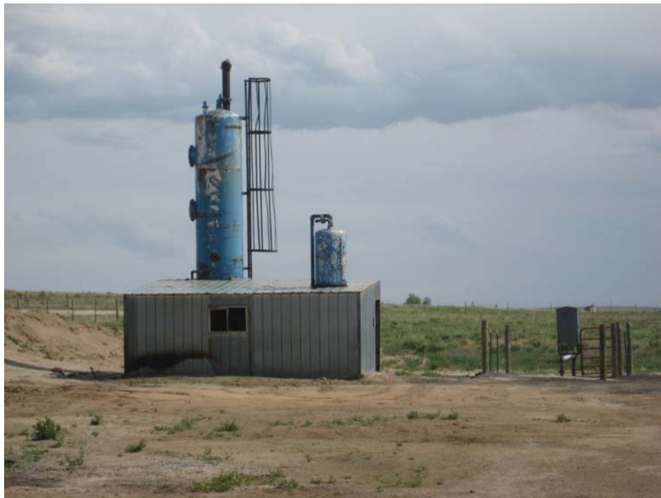
Photo 2. Separator on battery site for Myers 32-3 2
