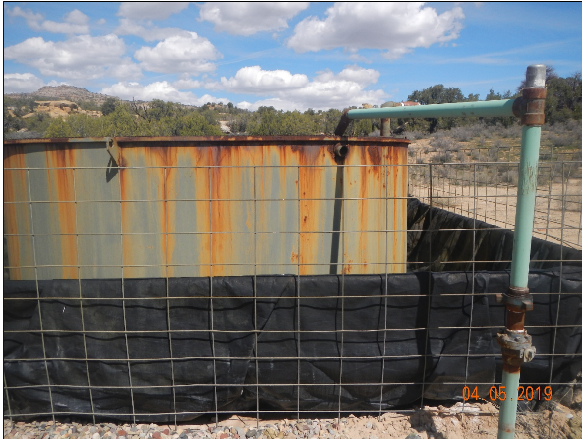
Photo #4 Tank need paint and has a lot of rust.
