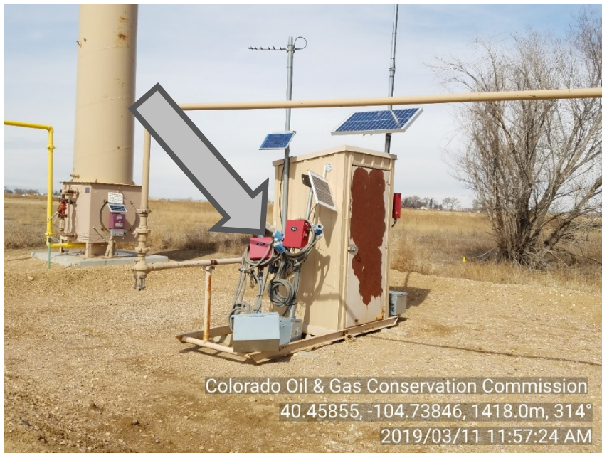
Photo #3 Weber 1-26 Gas meter run Unused Equipment - Automation controls from prior FIR
