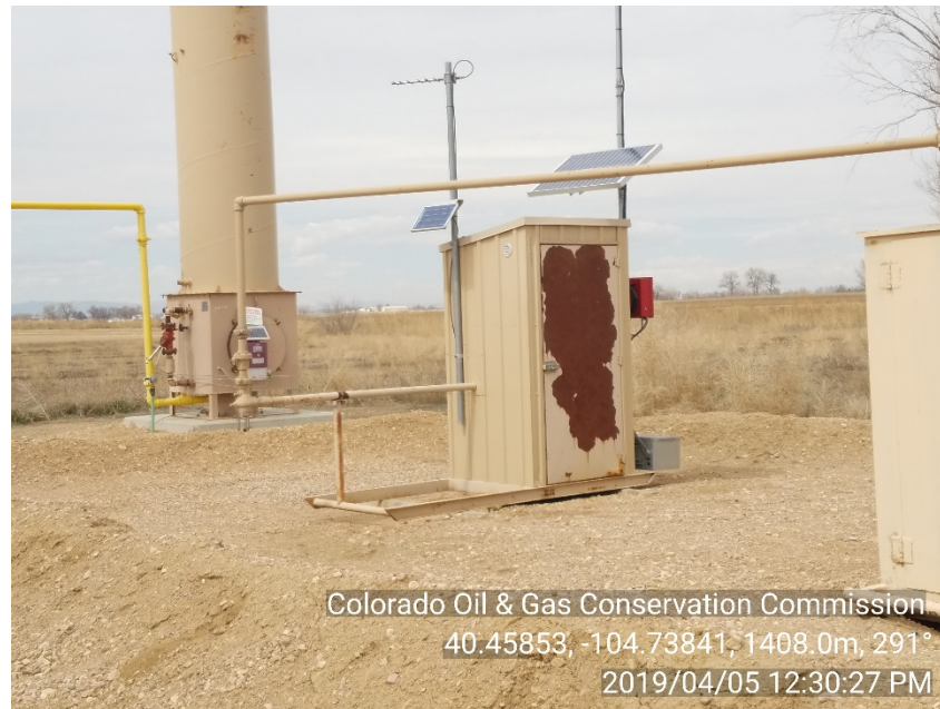
Photo #4 Weber 1-26 Gas meter run Unused Equipment - Automation controls Removed
