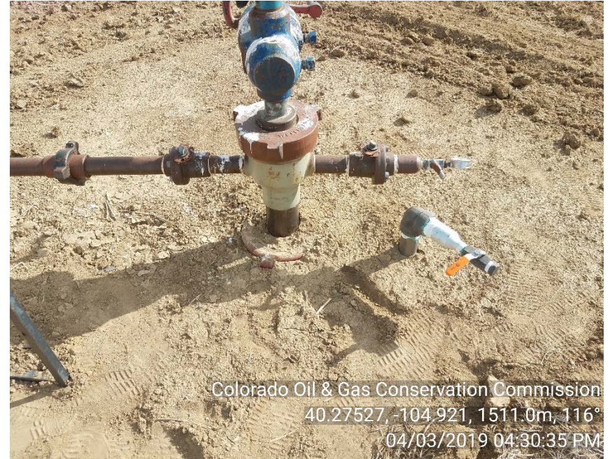
Bradenhead valve on 4/3/19
