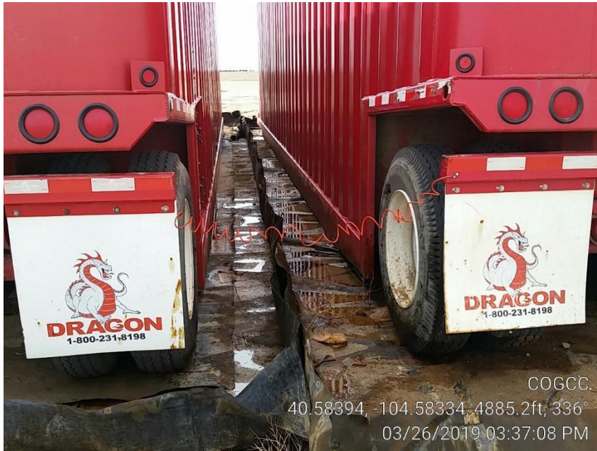
Photo 3 – Flowback Tanks have been grounded and bonded
