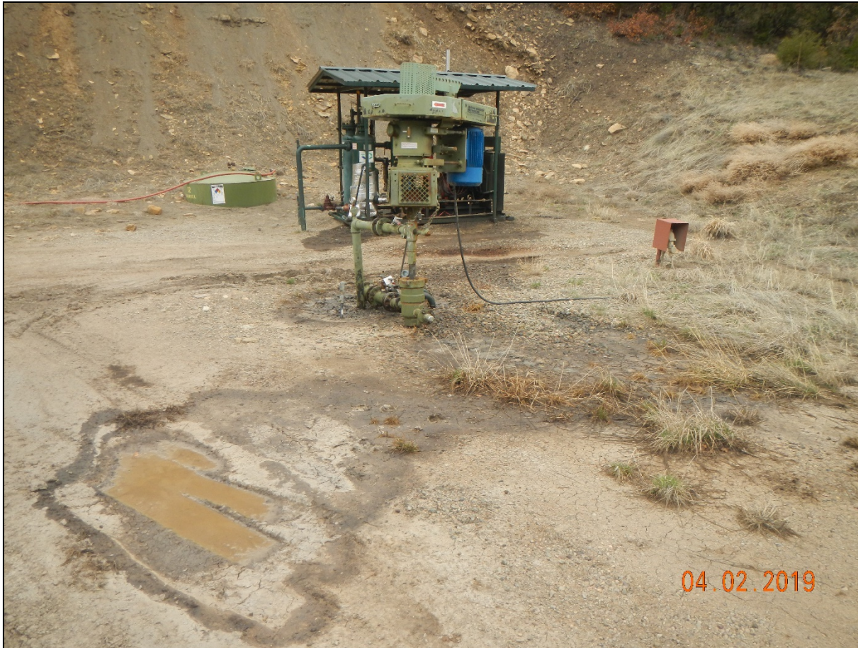
Photo 1. Facing toward the wellhead. It appears there was leakage.
