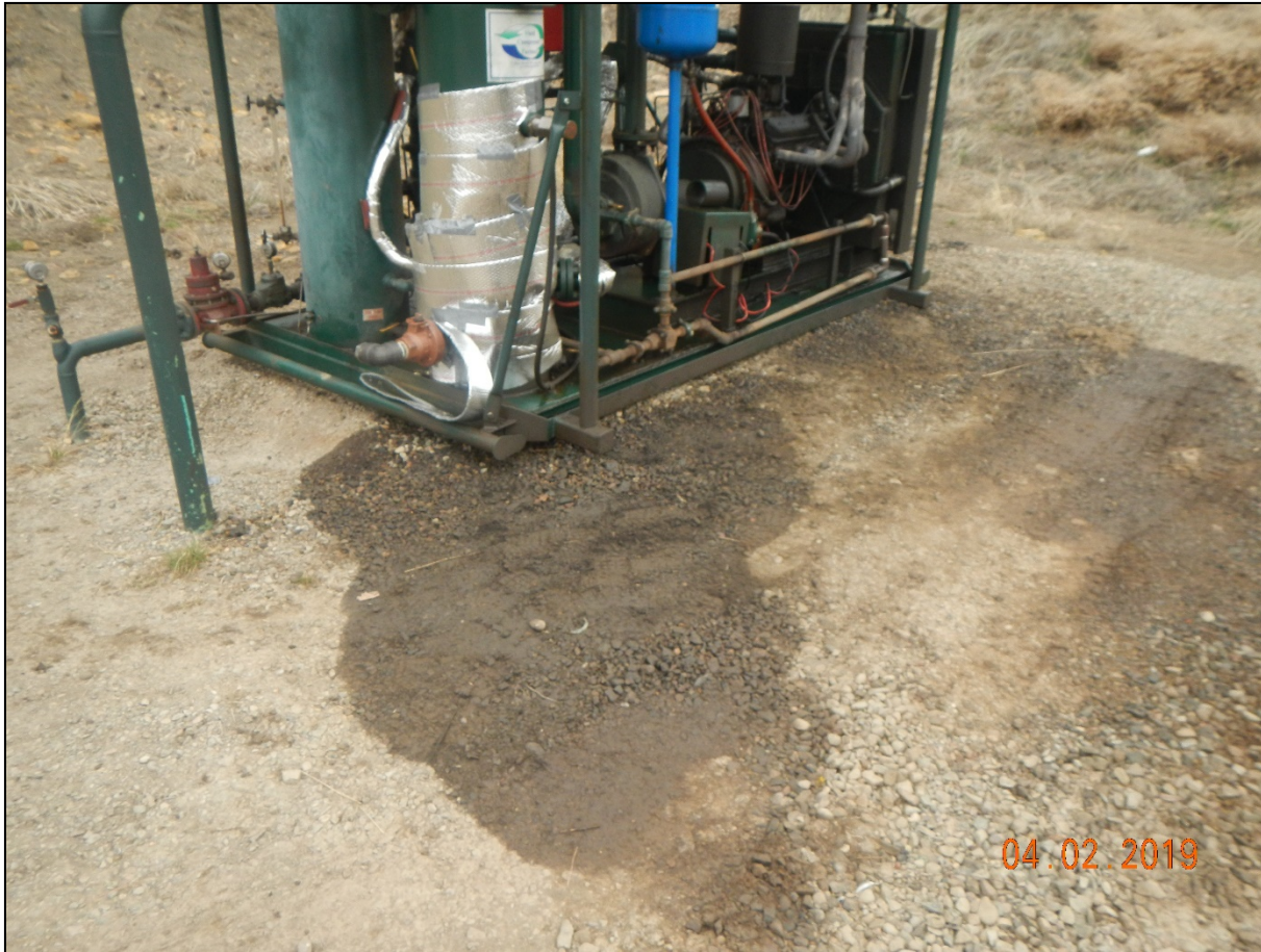
Photo 2. There is stained soil near the engine skid.
