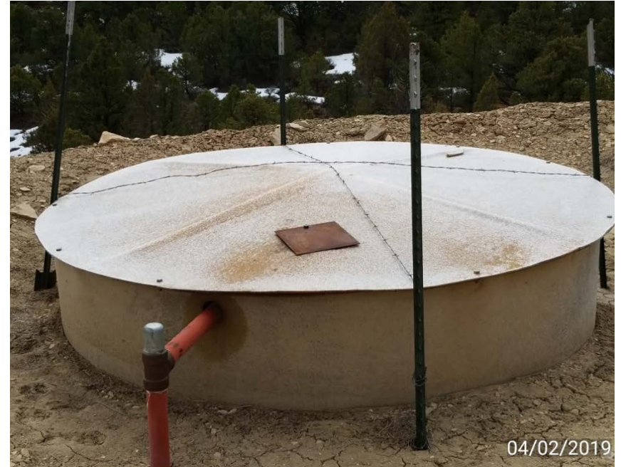
Photo 4. No tank sign.
