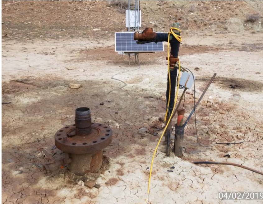
Photo 3. No well head sign.
