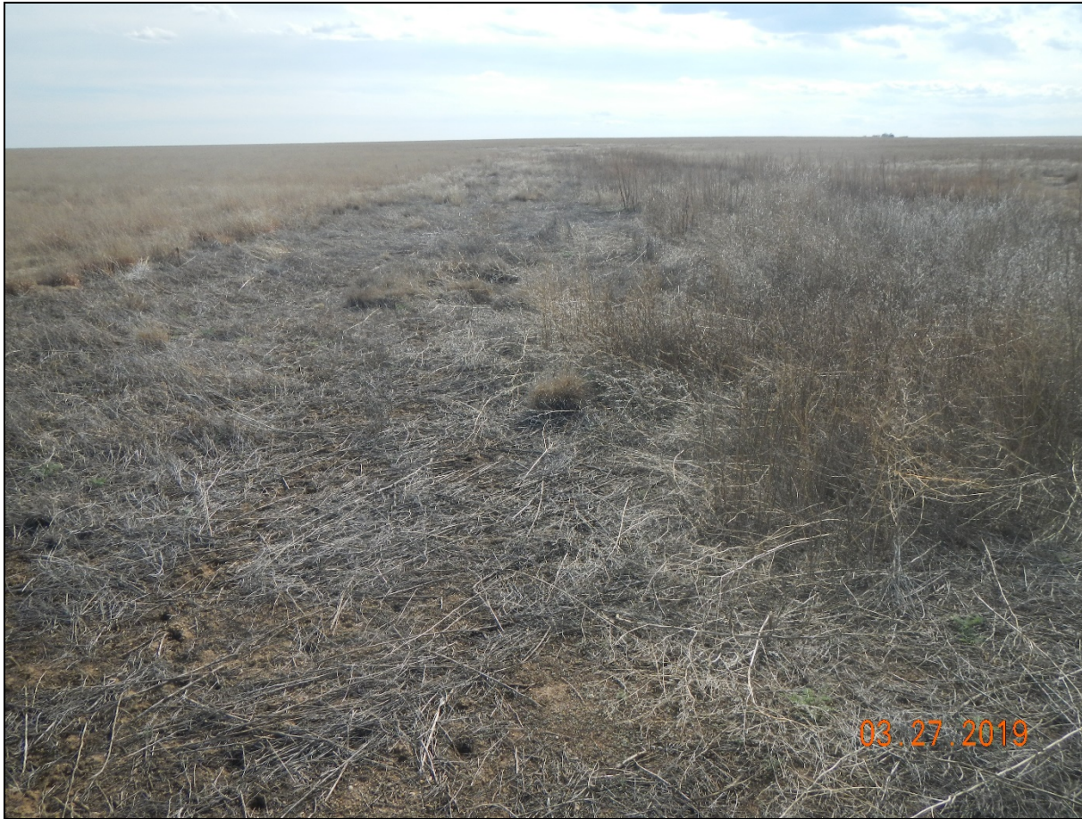
Photo 2. Facing southwest at the beginning of the access road. There are undesirable weeds along the road and desirable vegetation has not established.
