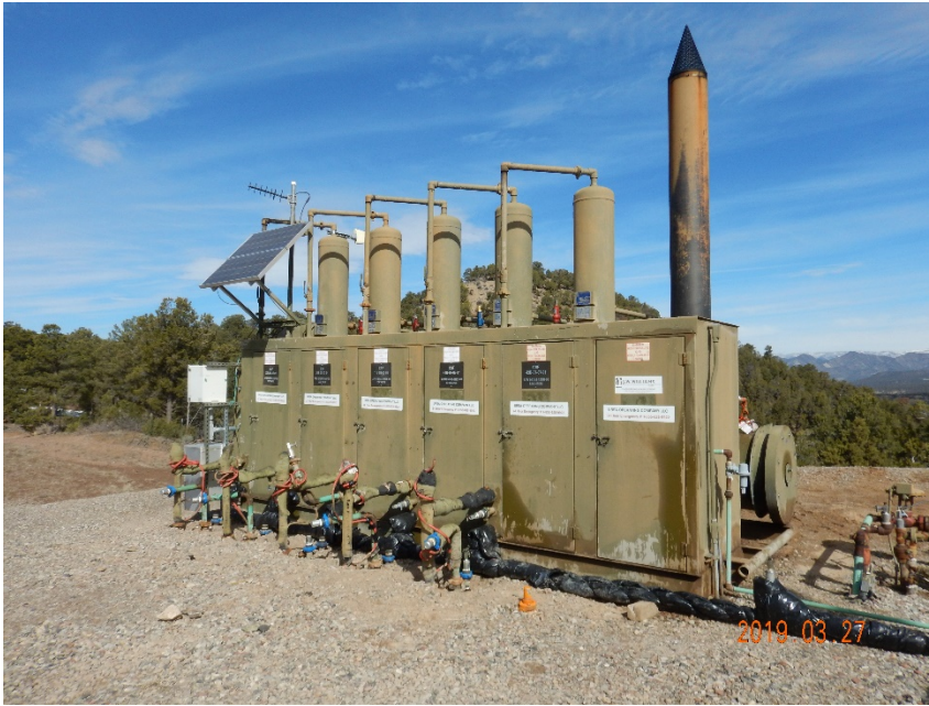
Photo #5 – View of vertical heated separators, looking north. Note that fired vessel on right side of this photo had been disconnected with components LOTO prior to inspection date.
