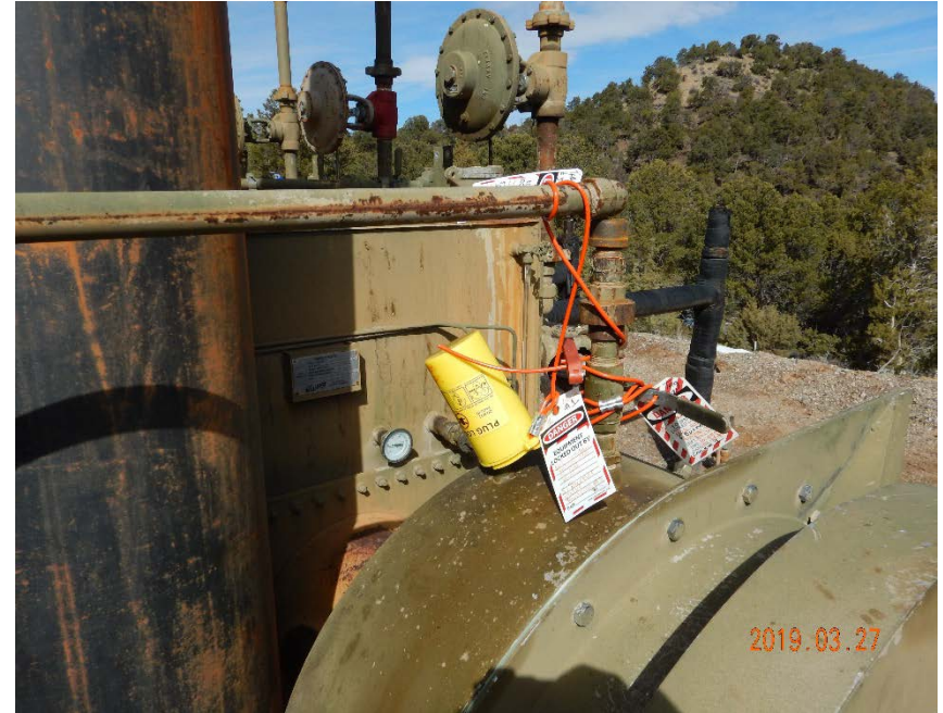
Photo #6 – LOTO components of fired vessel from previous photo.
