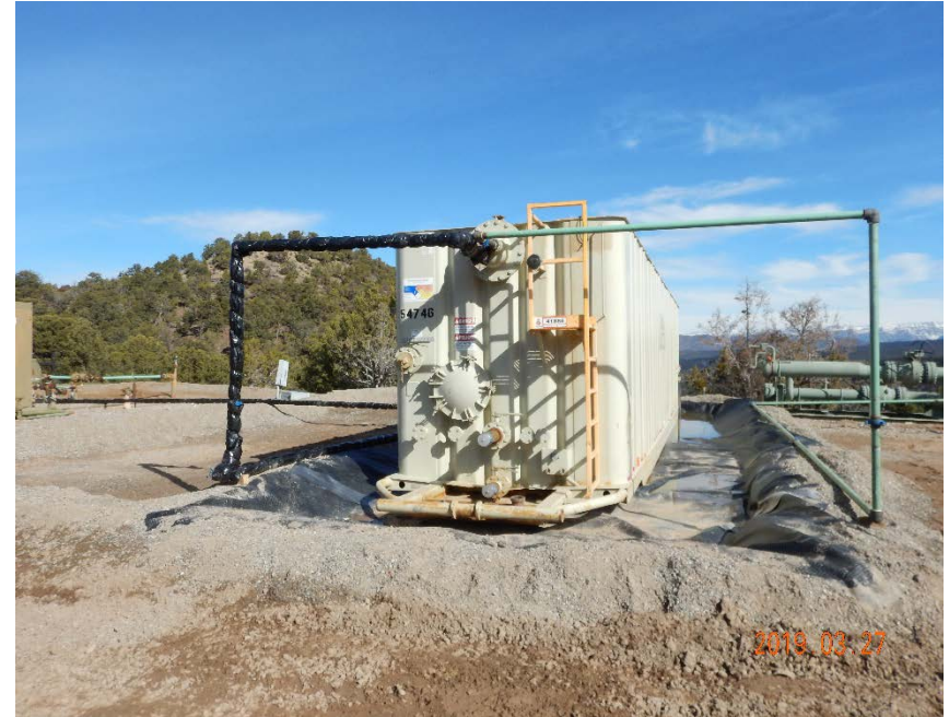
Photo #4 – View of temporary tank battery (looking north): 500 bbl frac tank in lined secondary containment.
