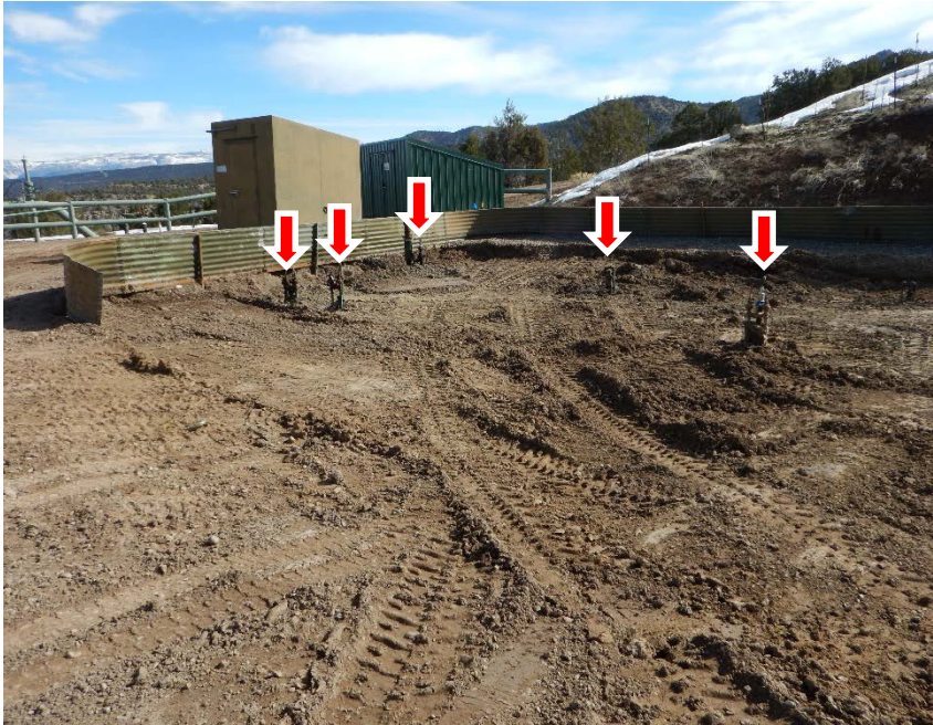
Photo #1 – View of deconstructed former tank battery, looking northeast. Note presence of flowline risers within former containment area (red arrows).
