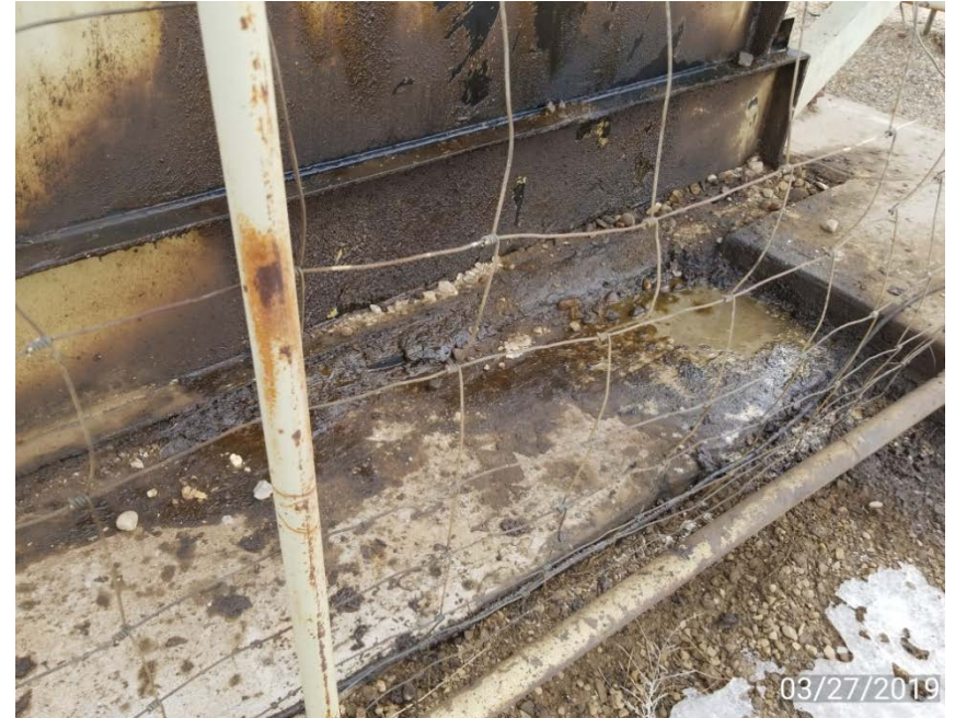
Photo 2. Oily waste on ground.
