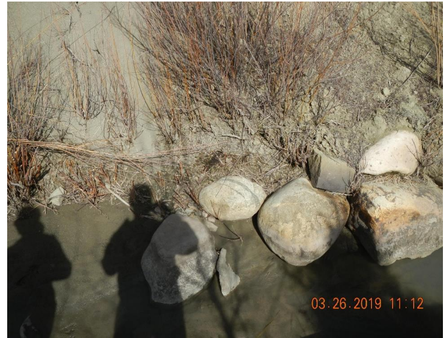
Impacted soil and vegetation remain along High Flume siphon bypass.
