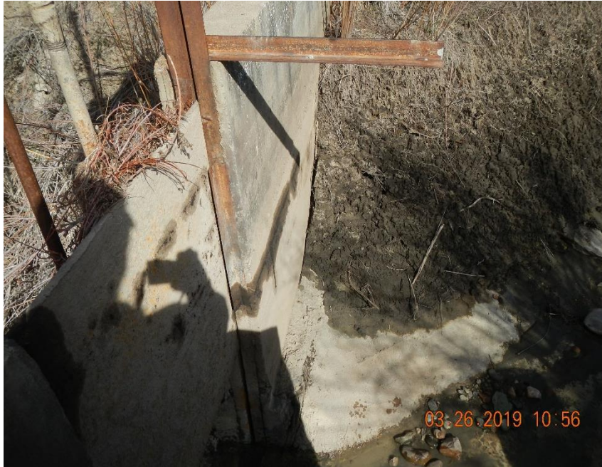
Stained concrete adjacent to High Flume siphon bypass.
