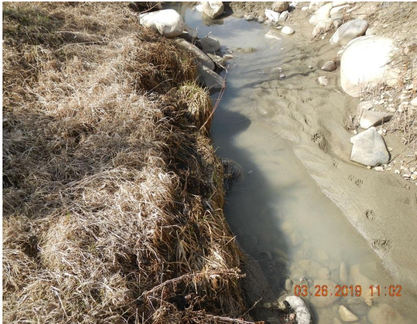
Impacted soil and vegetation along High Flume siphon bypass.
