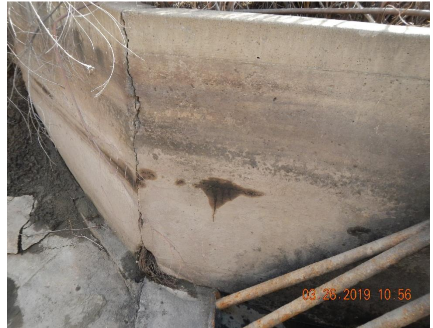
Oil stained concrete at High Flume siphon inlet.
