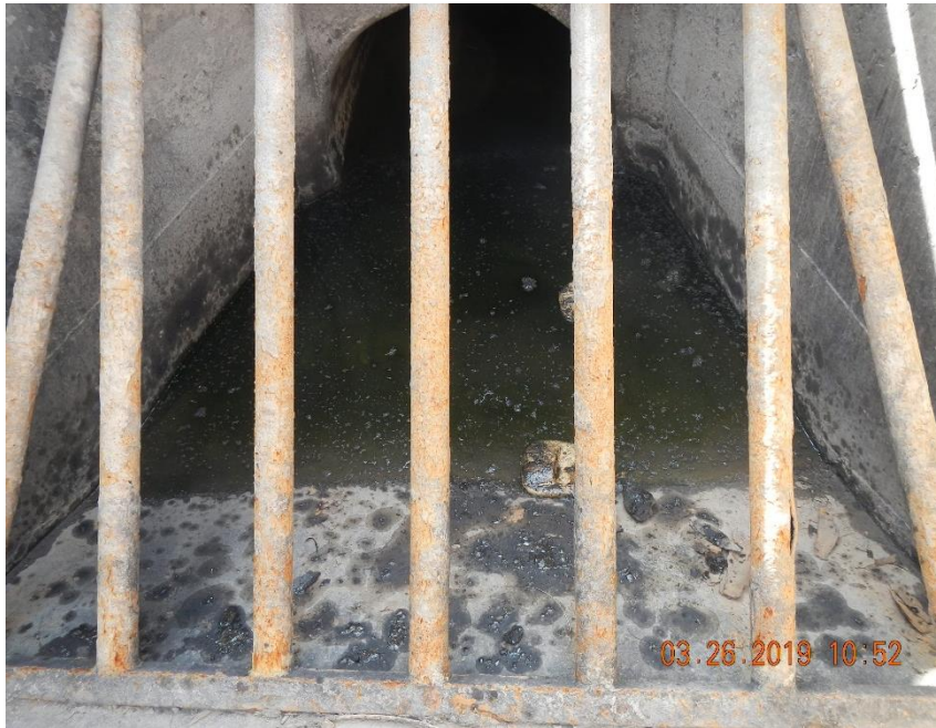
High Flume siphon inlet with residual E and P waste.
