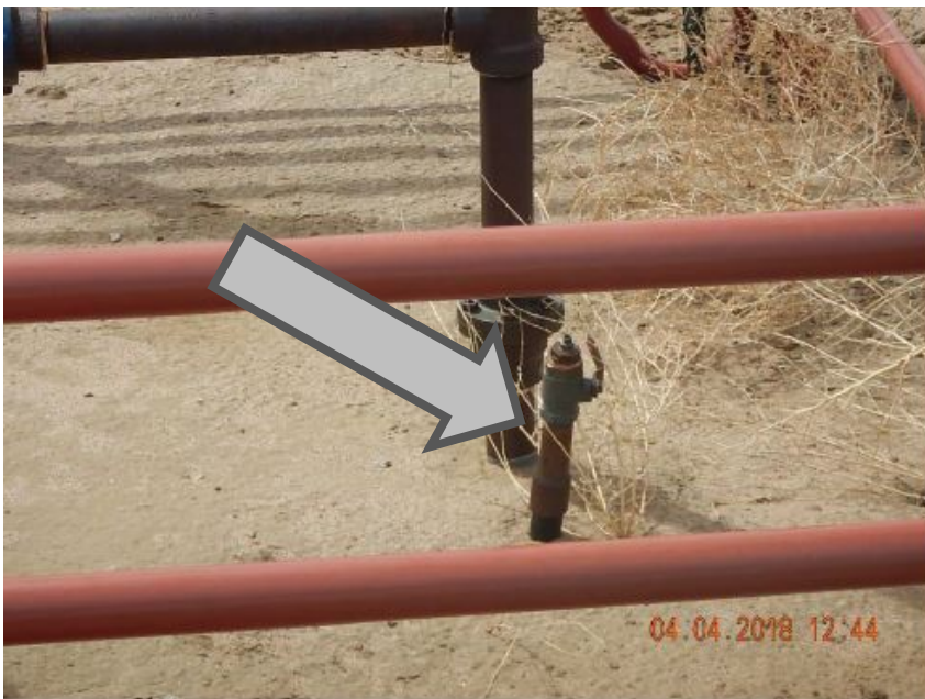
Photo #3 State 23-32 Wellsite Unused riser from prior FIR
