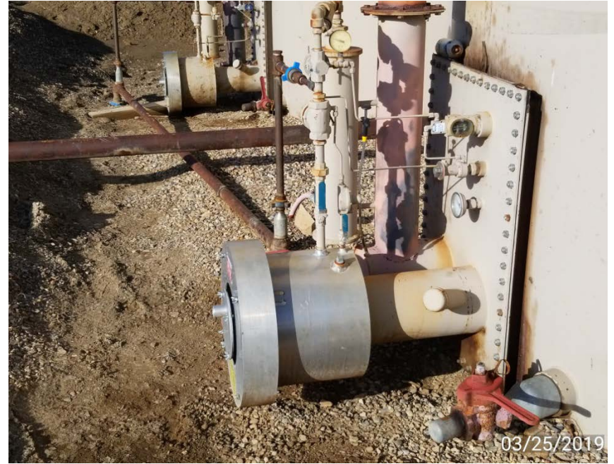
Photo 4. Tank battery burners.
