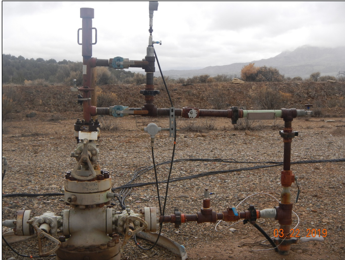
Photo of Wellhead
