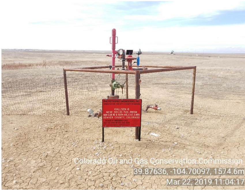
Photo 1 WH Kim Ray vlv appears to have been repaired
