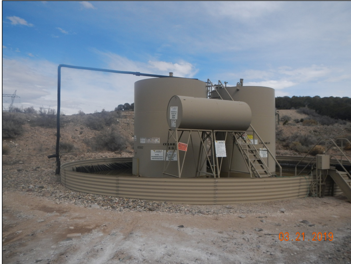
Photo of Tank Battery
