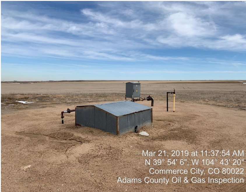
Photo#3 Gas Meter/Header Valve Shack
