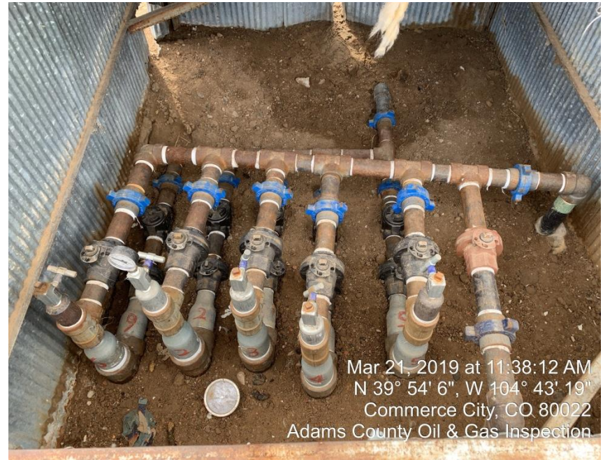
Photo#4 Inside Header Valve Shack
