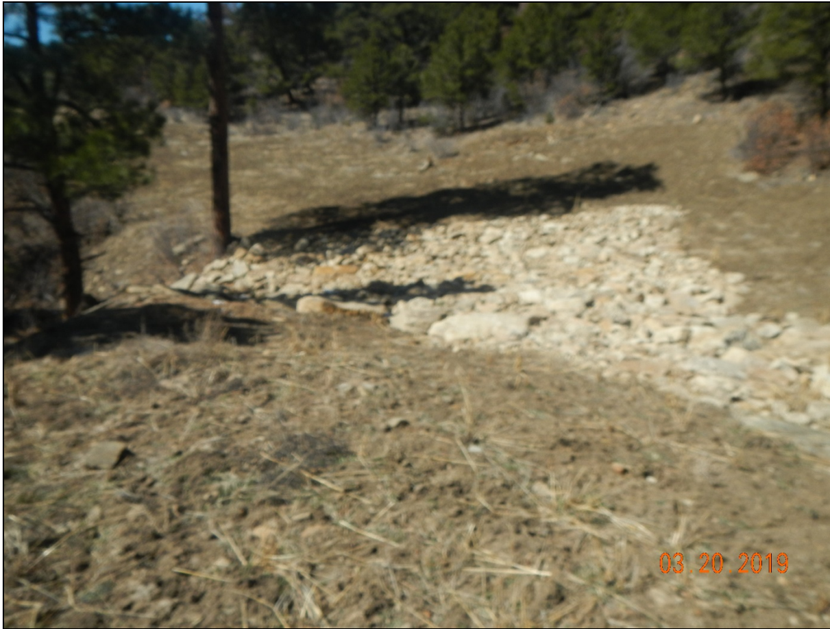
Photo 1. Facing toward the beginning of the reclaimed access road. Rock rip/rap has been placed in the drainage channel for erosion control.
