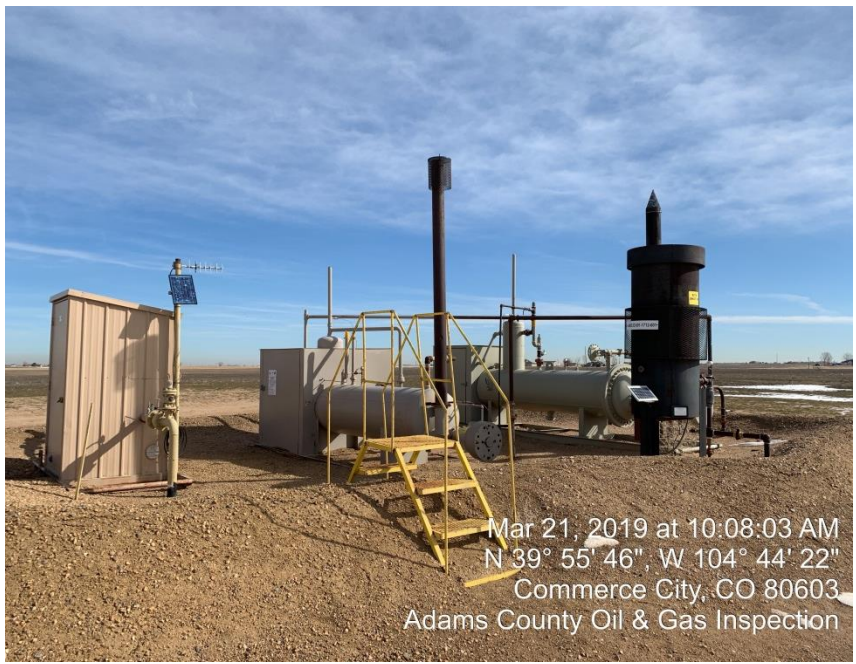
Photo#2 Gas Meter/(2)Separators/ECD
