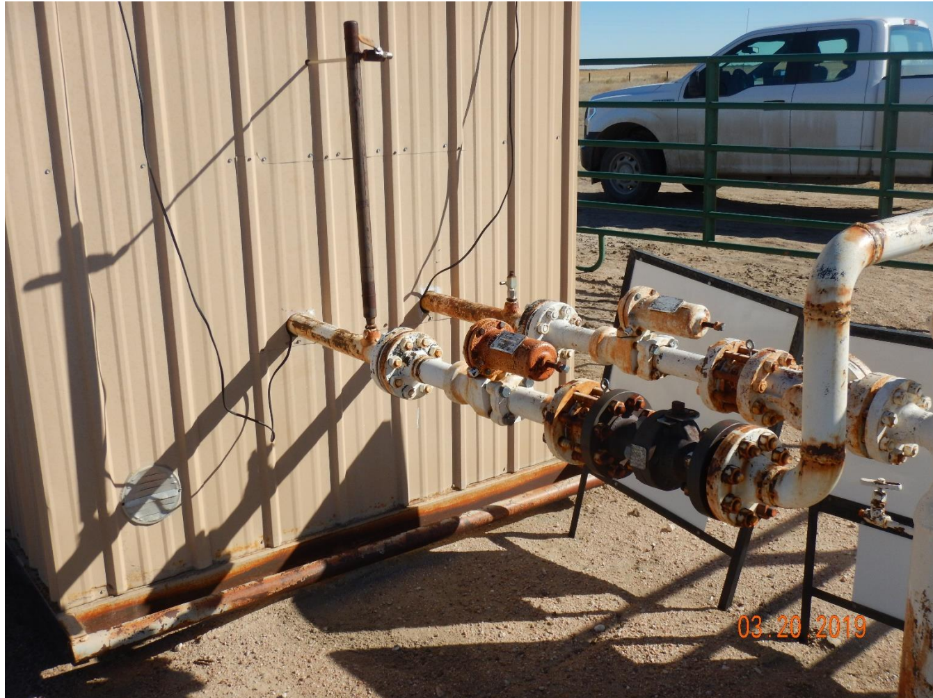
Photo 3: Continued from photo 2. Photo shows lines behind “Rosewood” signs.
