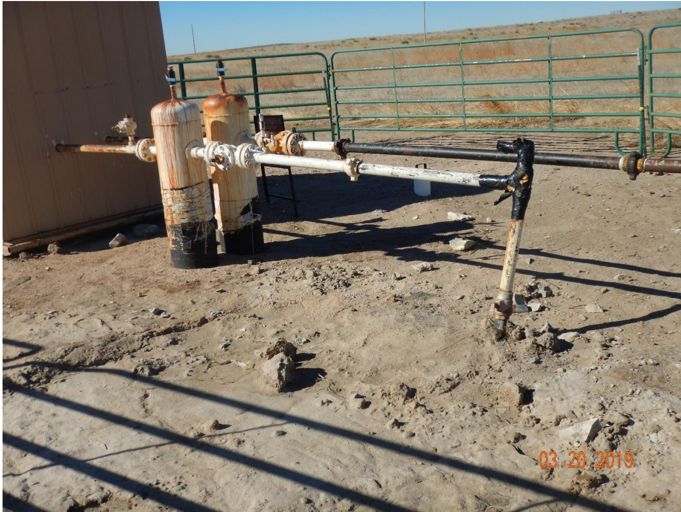
Photo 4: Photo taken from the north end of the equipment. Photo of lines/equipment.
