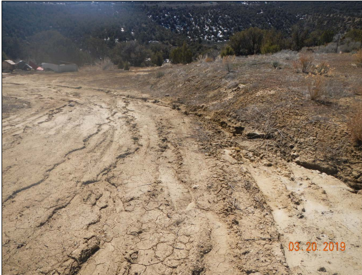
Storm water erosion not to being controlled on the location at this time.
