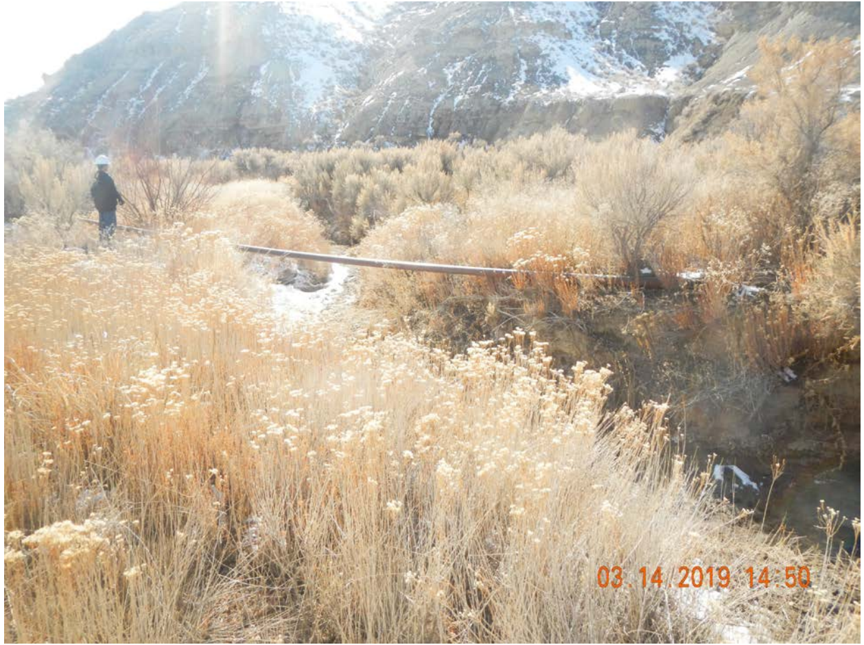
Flowline that was crossing part of Vermillion Creek.
