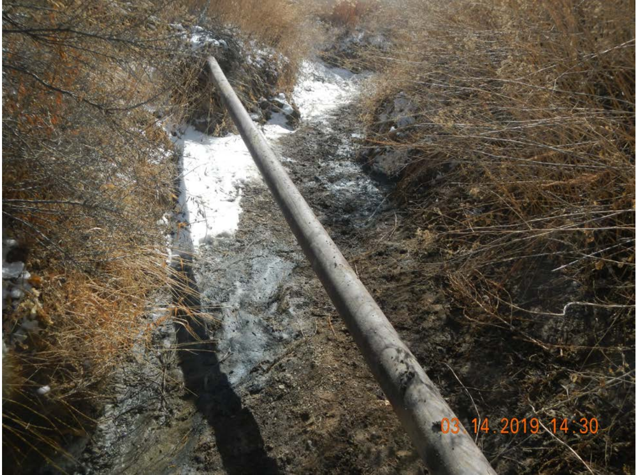
Flowline crossing creek bed.
