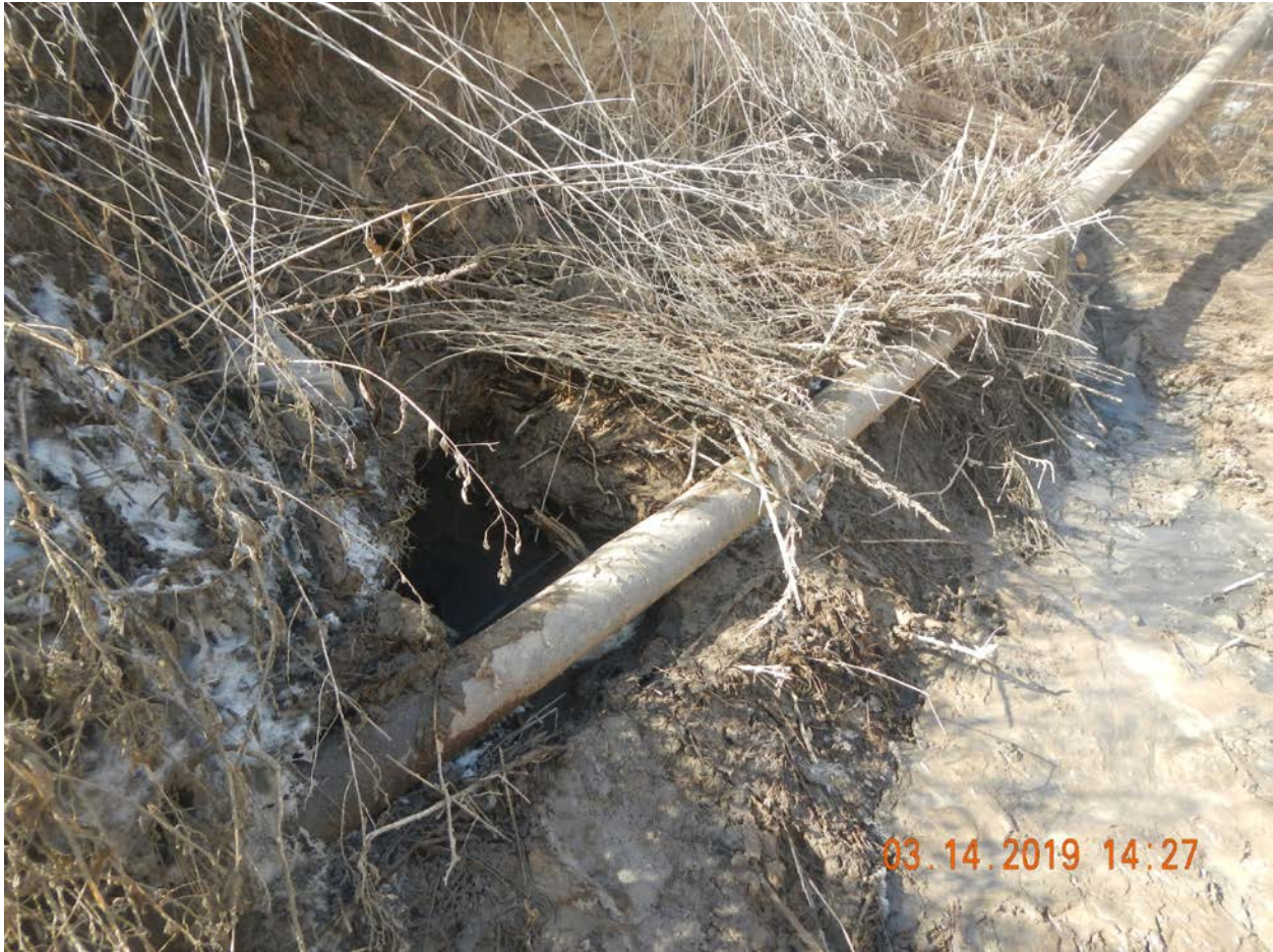
Spill Point, note area of erosion, the pipe failed on the underside forcing fluid to erode the side bank of creek.
