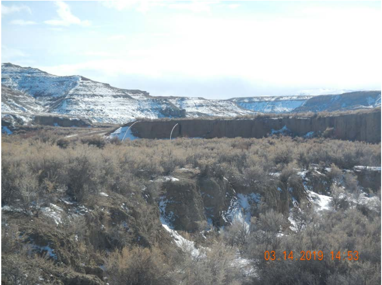
Note: two flowlines coming out of hillside. It was reported that the failed line is the one on left of photo.
