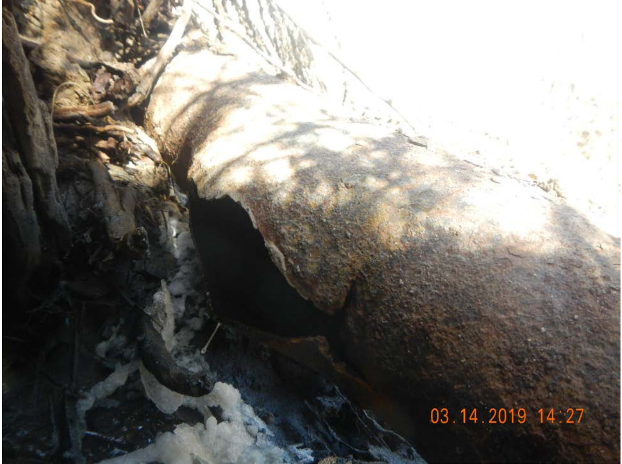
Spill point, pipe failure.
