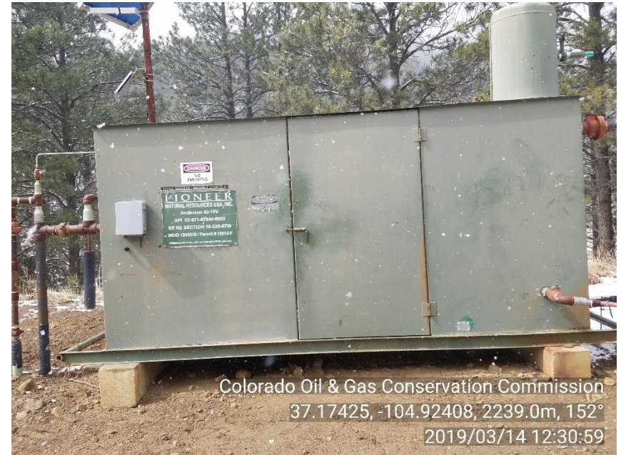
PHOTO 2: WELL SIGN/METER HOUSE
