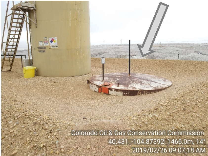
Photo #3 Knox 32-3 Unmarked Tank Contents / Capacity NOT posted from prior FIR
