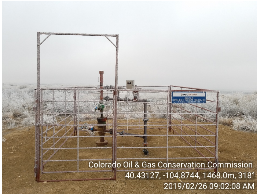
Photo #1 Knox 32-3 (05-123-20645) Wellsite Shut-In | SI – LOTO from prior FIR
