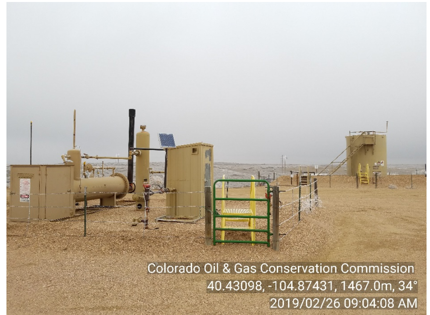
Photo #2 Knox 32-3 Battery Shut-down from prior FIR
