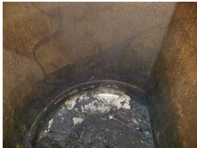
Photo 4: Inside of vertical heater 1 treater after cleaning.
