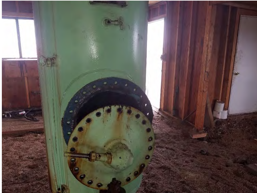
Photo 5: Vertical heater 2 treater in building.
