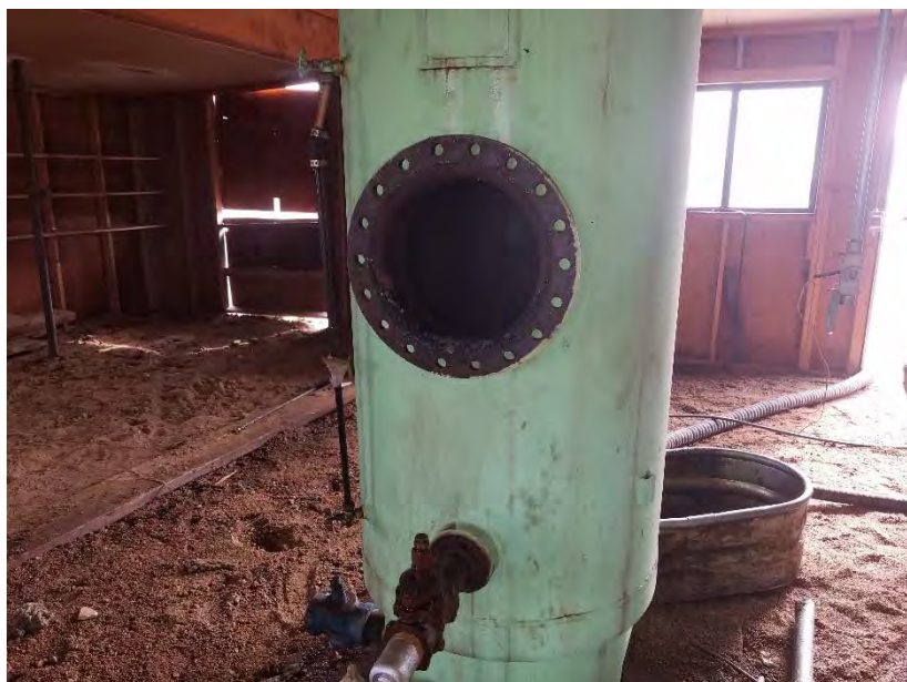
Photo 3: Vertical heater 1 treater in building.
