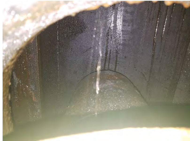
Photo 6: Inside of vertical heater 2 treater after cleaning.
