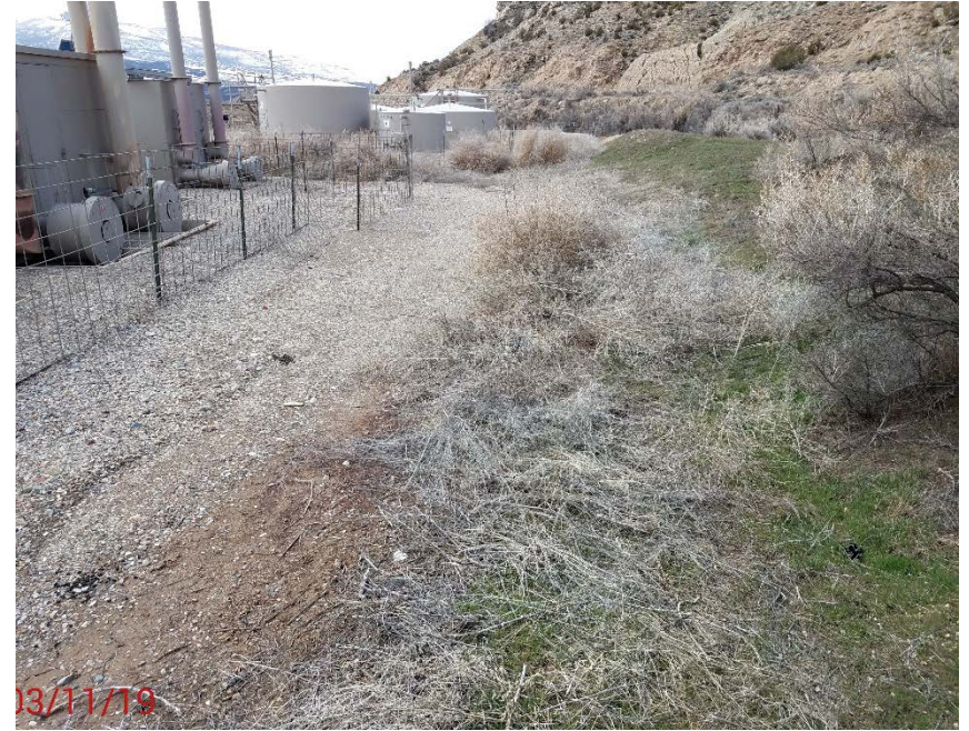
Location Photo #4, Debris behind the separators.
