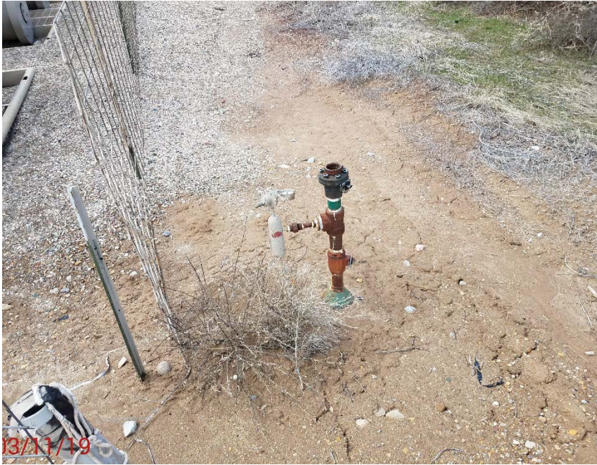
Location Photo #3, unmarked flowline.
