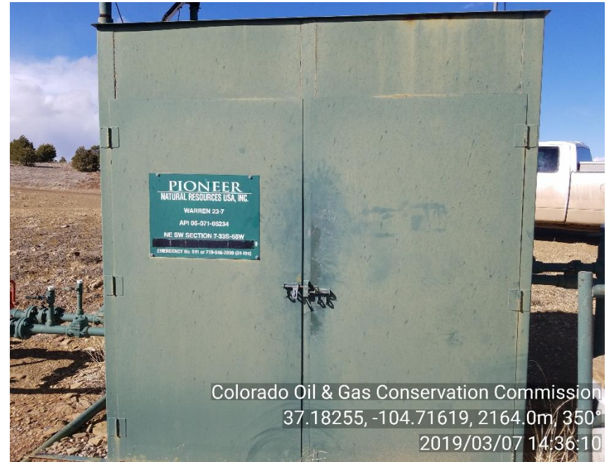
PHOTO 2: WELL SIGN/METER HOUSE
