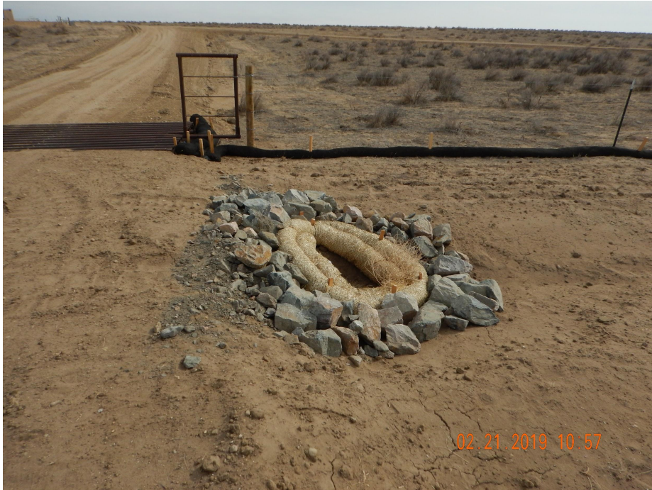
Photo 2. Photo taken from the northeastern entrance to location, facing East. Photo illustrates outlet protection for a culvert installed in conjunction with a ditch and berm which is directed to a retention area.
