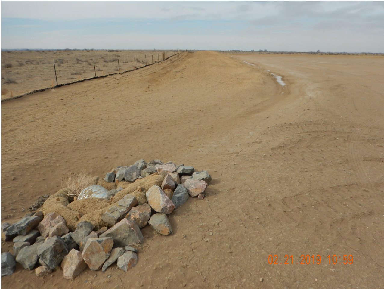
Photo 6. Photo taken from the southeastern well pad, facing West. Photo illustrates the southern topsoil stockpile- see comments under Photo 1. Photo also illustrates the ditch and berm BMP with a stabilized inlet for the culvert which is directed to a retention area.
