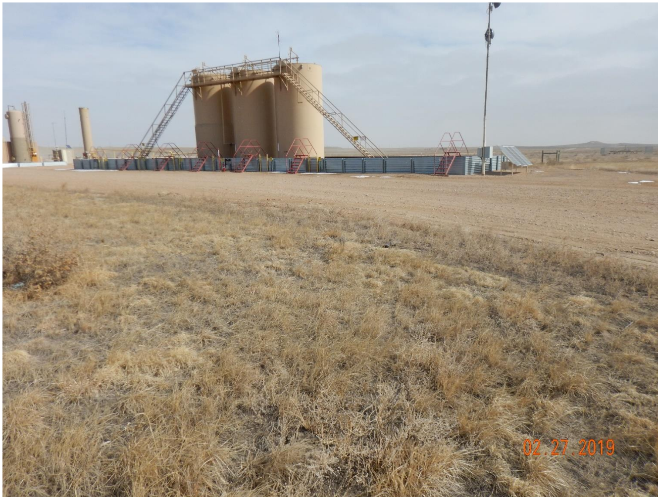
Photo 2: Photo taken from the location facing east. Location is abandoned. Photo shows no oil and gas disturbance appears to have been conducted.
