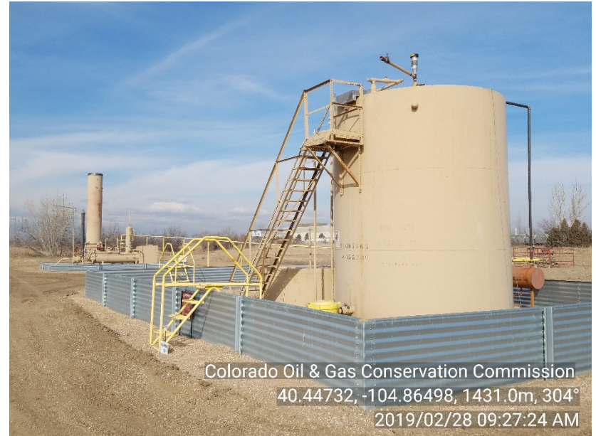
Photo #2 Great Western 35-52 Battery Shut-down
