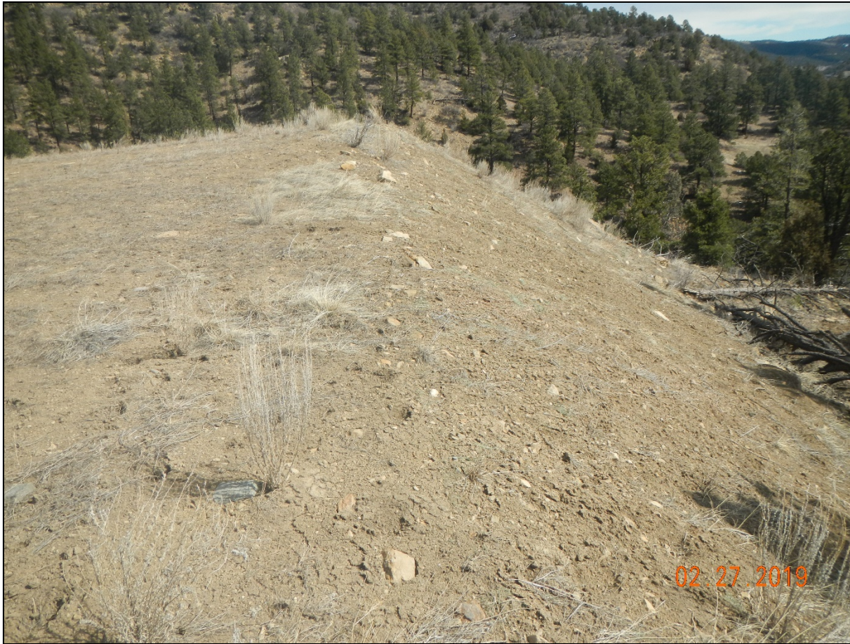
Photo 11. Facing east along the fill slope. Vegetation has not established along the fill slope which is susceptible to erosion.
