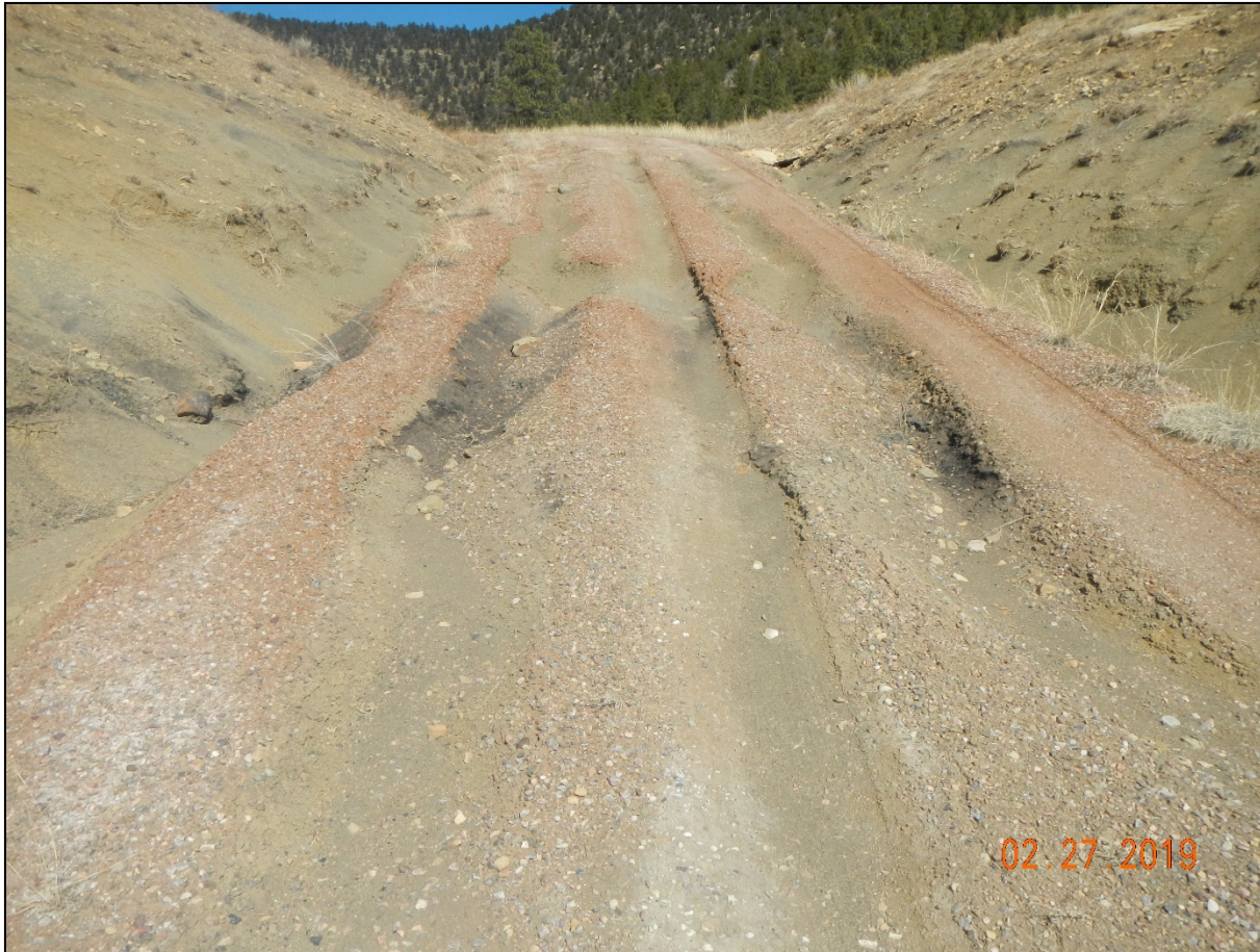
Photo 2. Erosion channels have developed on the access road
