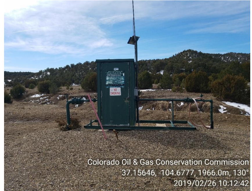
PHOTO 2: WELL SIGN/METER HOUSE/EMERGENCY CONTACT IS UPDATED.
