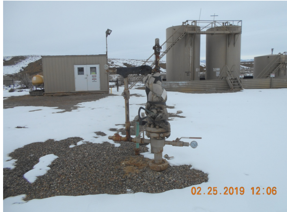
Wellhead , Pump Housing and Tank Battery
