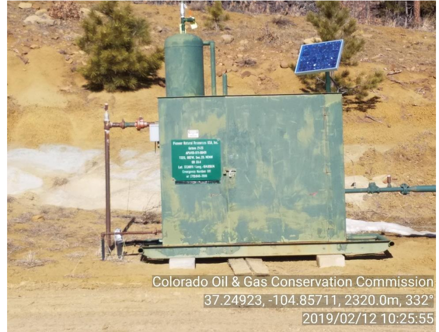
PHOTO 2: WELL SIGN/METER HOUSE
