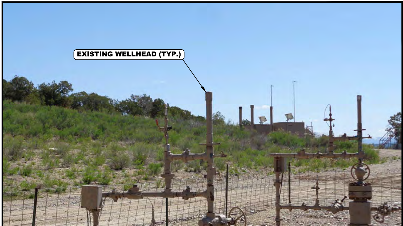
PHOTO: VIEW OF WELLHEADS
