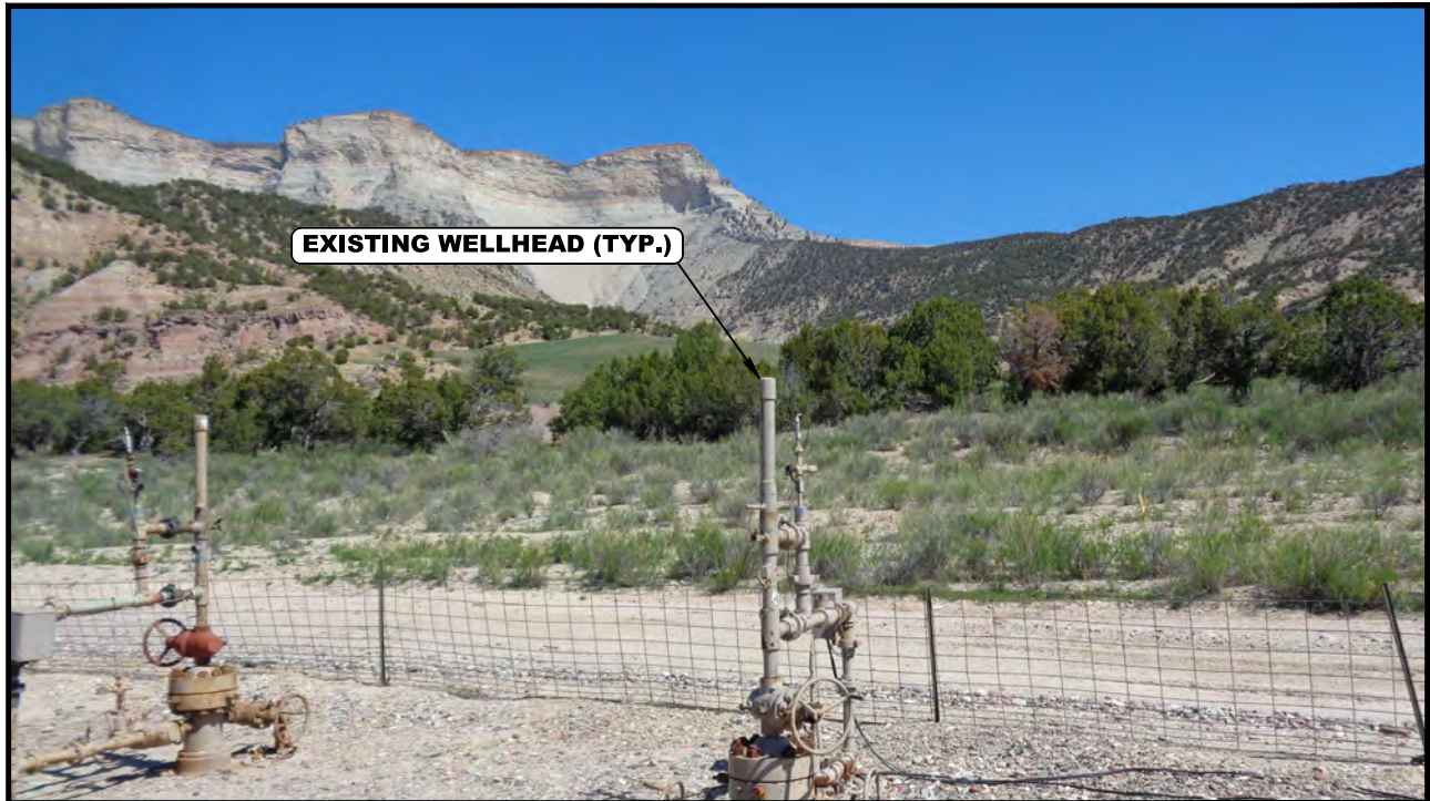
PHOTO: VIEW OF WELLHEADS
