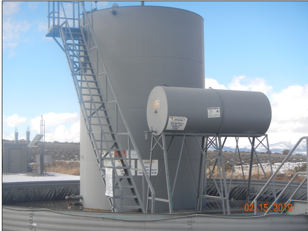
Tank Battery photo
