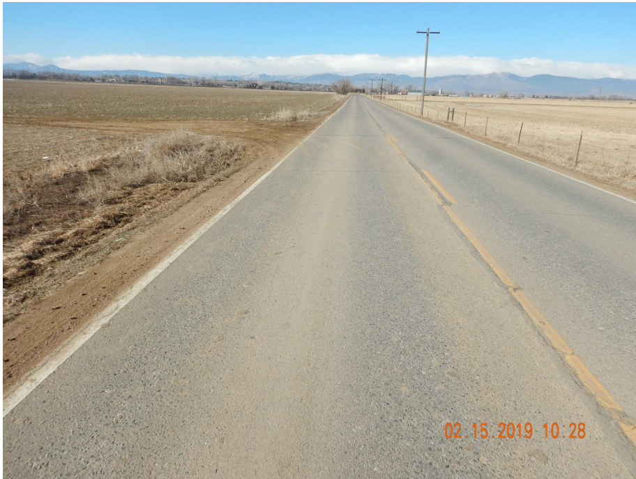
Photo 2. Photo taken from the entrance of the location off Niwot Rd. on 2/15/19, facing West. Photo illustrates no track out was observed at the time of this inspection. Operator dispatched a street sweeper to clean track out on 2/13.
