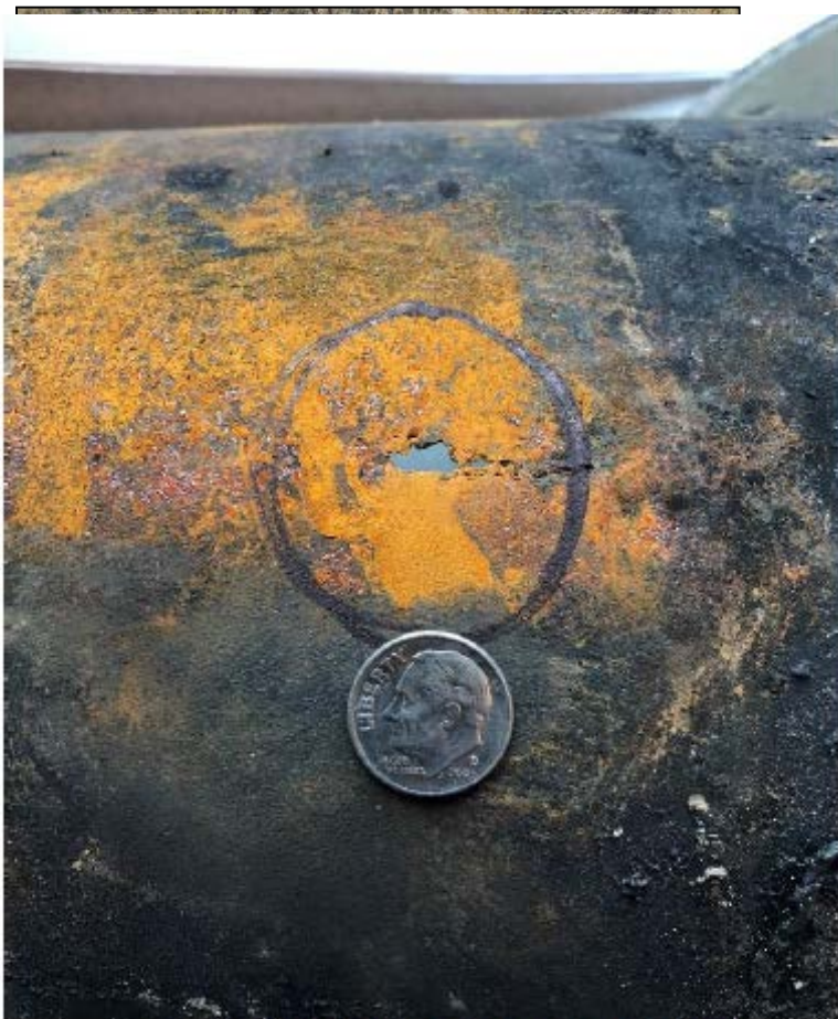
External View of Pipe Corrosion
