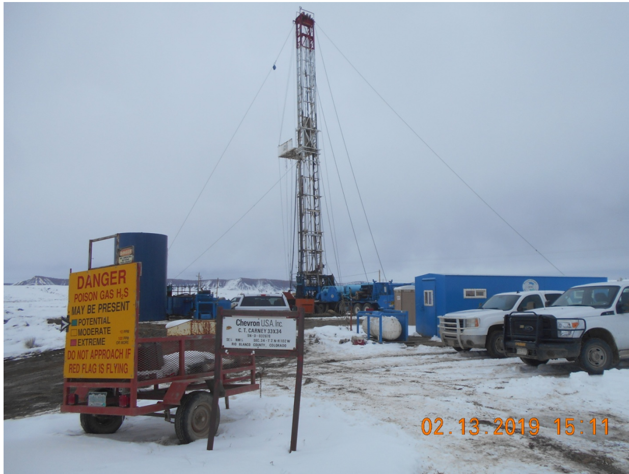
Workover rig on Injection Wellhead
