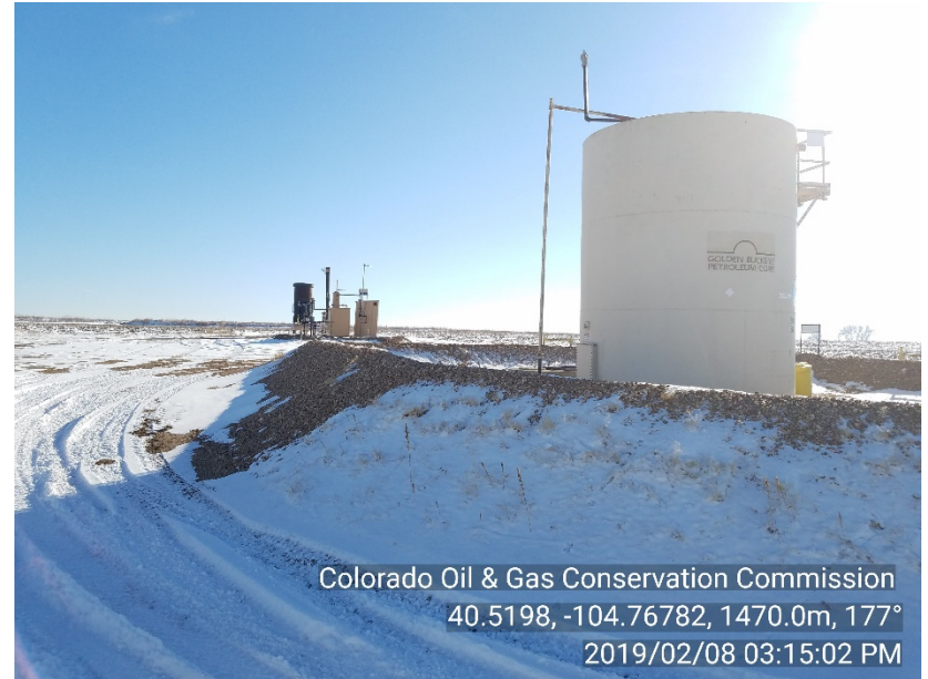
Photo #2 Sullivan 3-1 Battery Shut-Down
