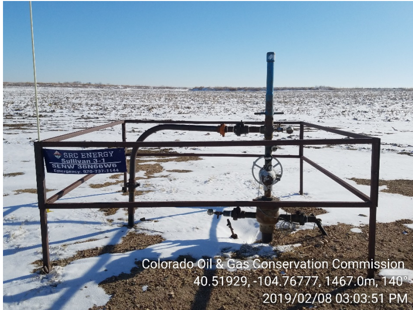
Photo #1 Sullivan 3-1 (05-123-12925) Wellsite Shut-In | SI
