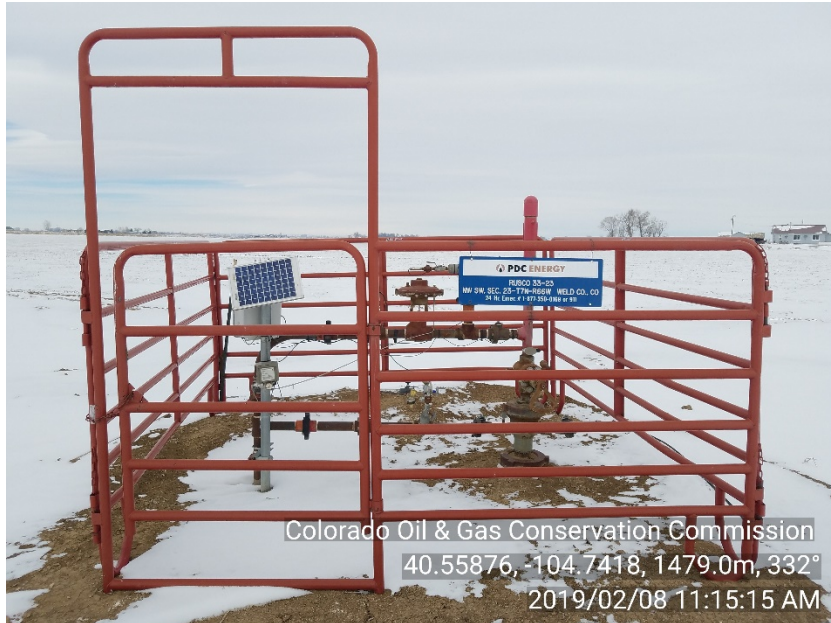
Photo #1 Rusco 33-23 (05-123-25026) Wellsite Shut-In | SI
