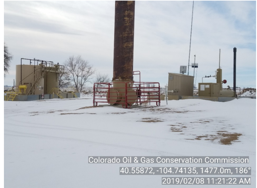
Photo #2 Rusco 33-23, 43-23 Battery Shut-down
