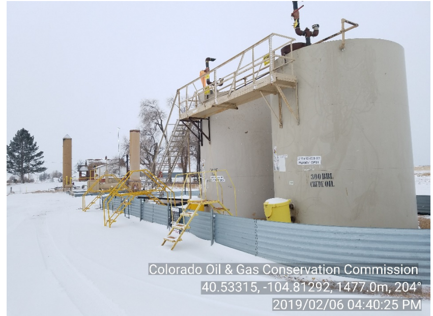
Photo #2 Deines 31-11, 31-14 Battery Shut-down
