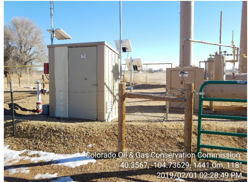
Photo #4 Schank J 35-7, 35-08, 35-17, 35-22 Unused / disconnected gas meter run Has been removed from site
