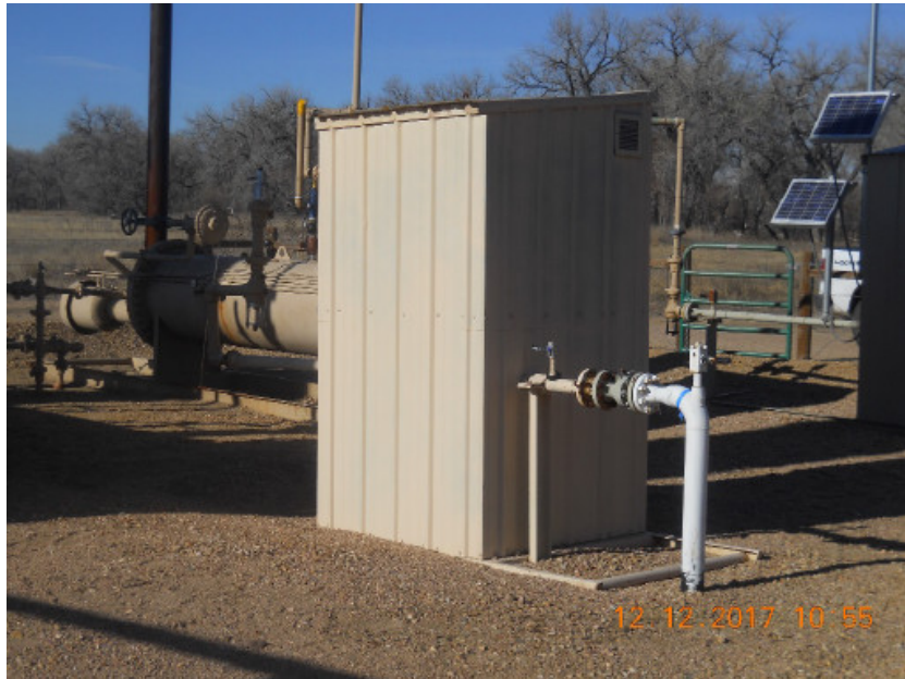
Photo #3 Schank J 35-7, 35-08, 35-17, 35-22 Unused / disconnected gas meter run from prev. FIR
