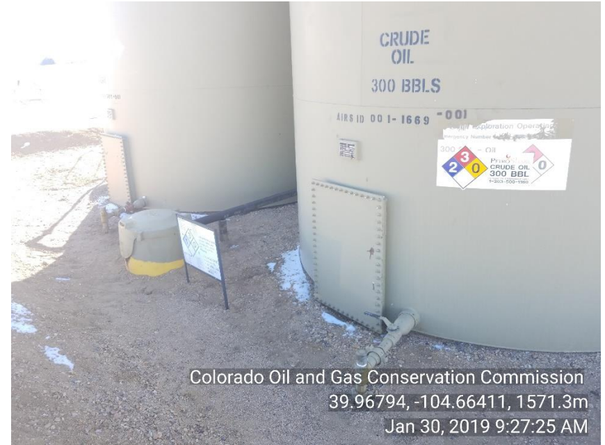
Photo 6 load lines in front of crude oil tanks
