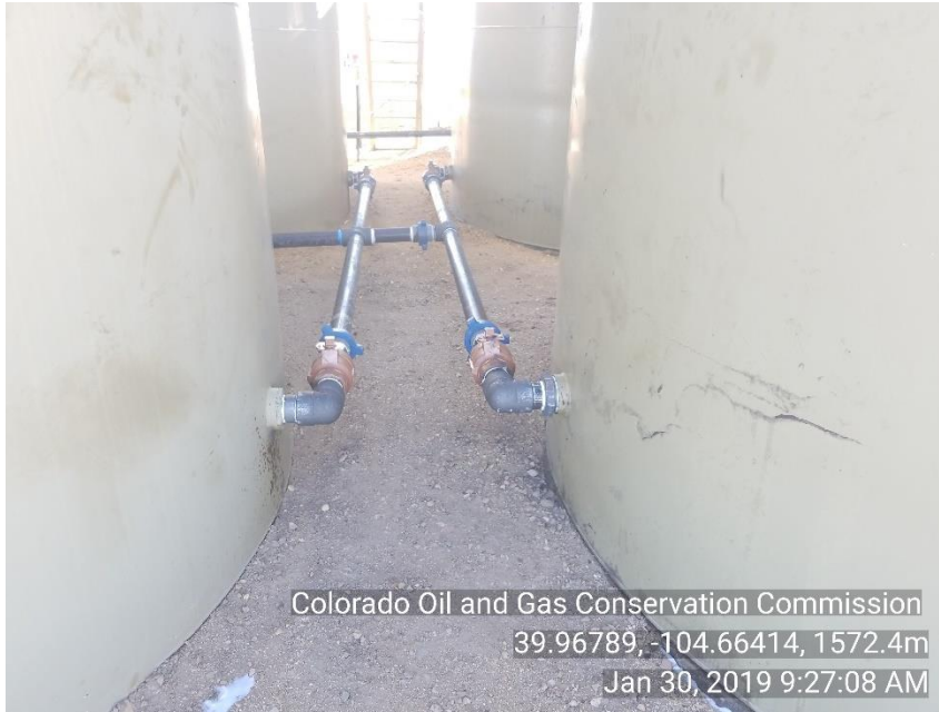
Photo 5 lines between crude oil tanks
