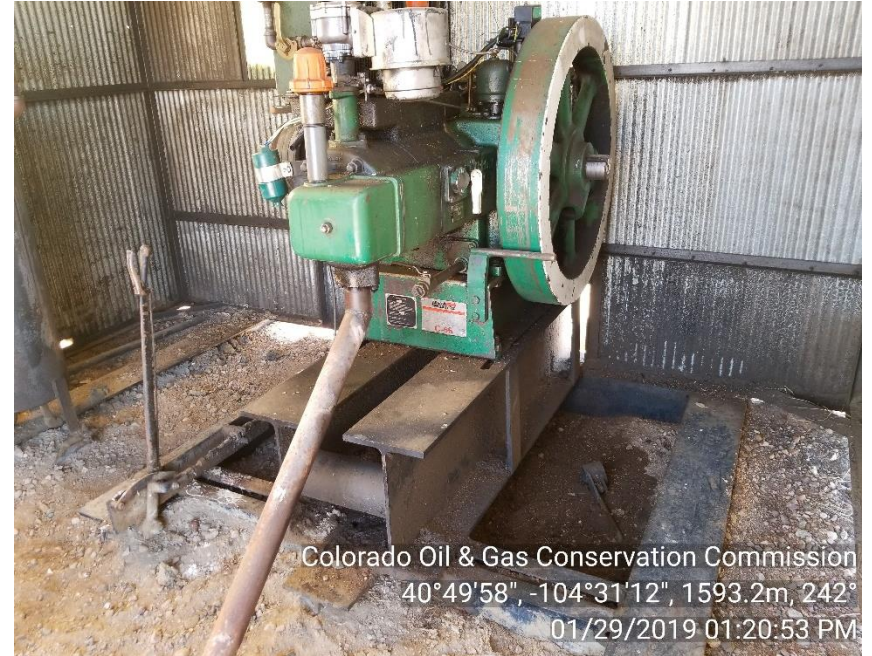
Photo 4: Stained soil under pump jack motor
