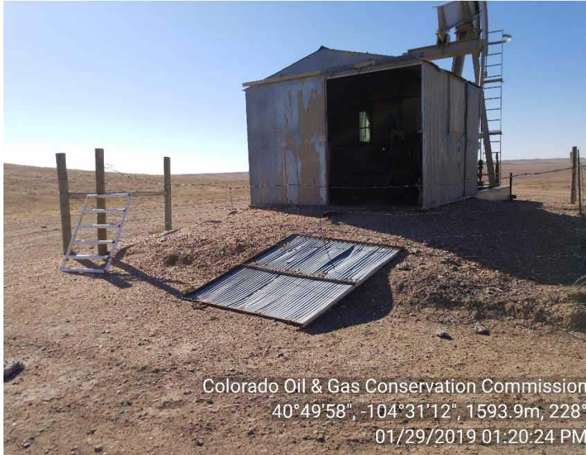
Photo 3: Door from pump jack shed and gate to fencing in disrepair.
