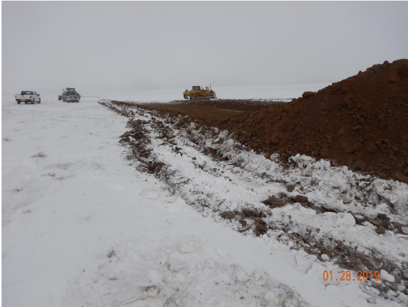
Photo 1: Photo taken from the southwest end of the location, facing north. Photo shows topsoil salvage and pad construction in process. Photo also shows operator has installed surface roughening along the perimeter of the location.
