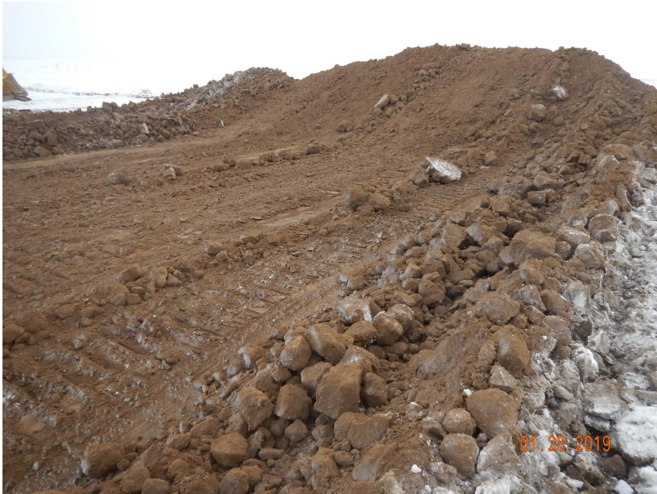
Photo 4: Photo taken from the south end of the location, facing south. Photo of topsoil salvage in process.
