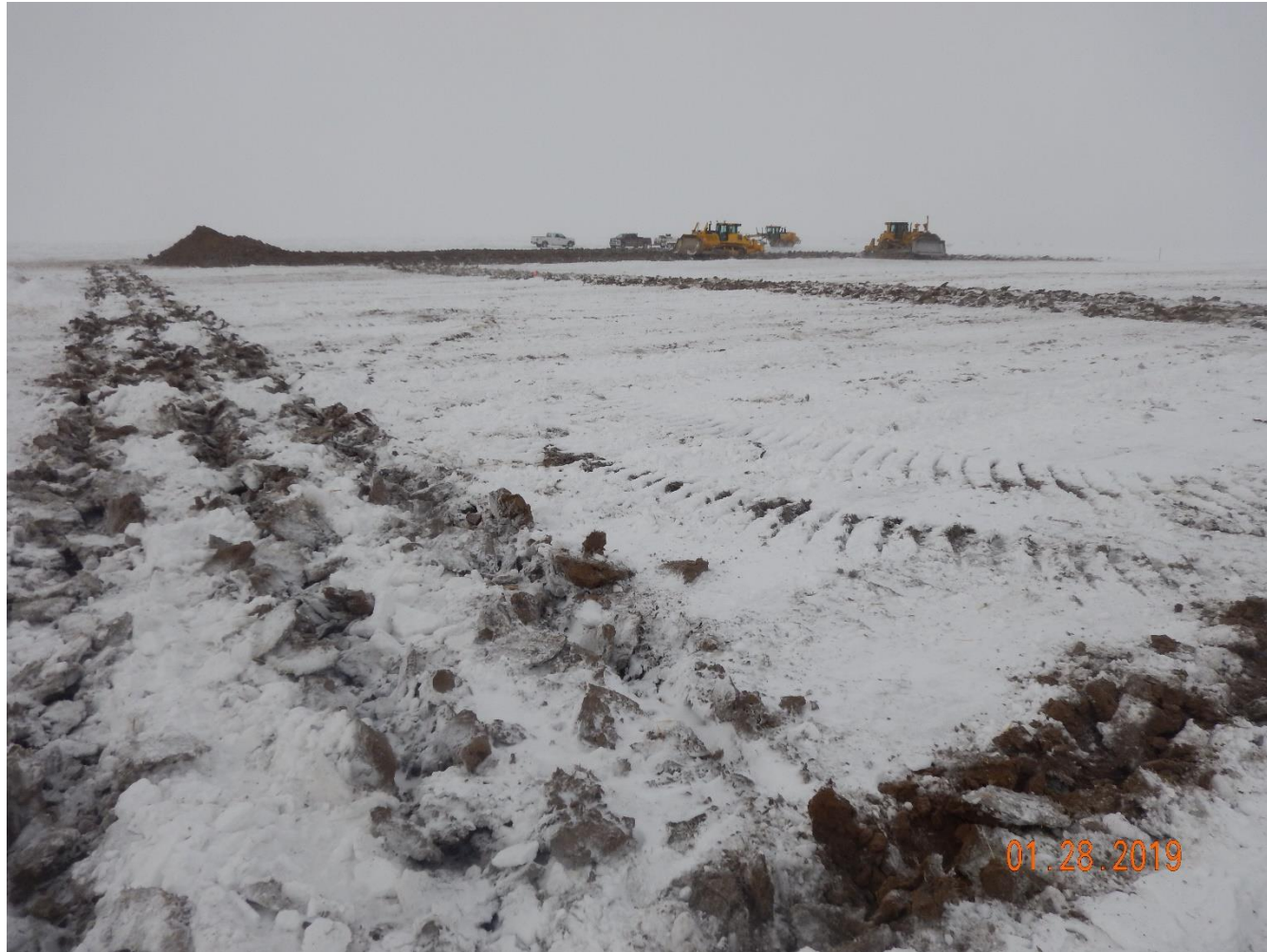
Photo 3: Photo taken from the southeast end of the location, facing northwest. Photo shows topsoil salvage and pad construction in process. Photo also shows operator has installed surface roughening along the perimeter of the location.
