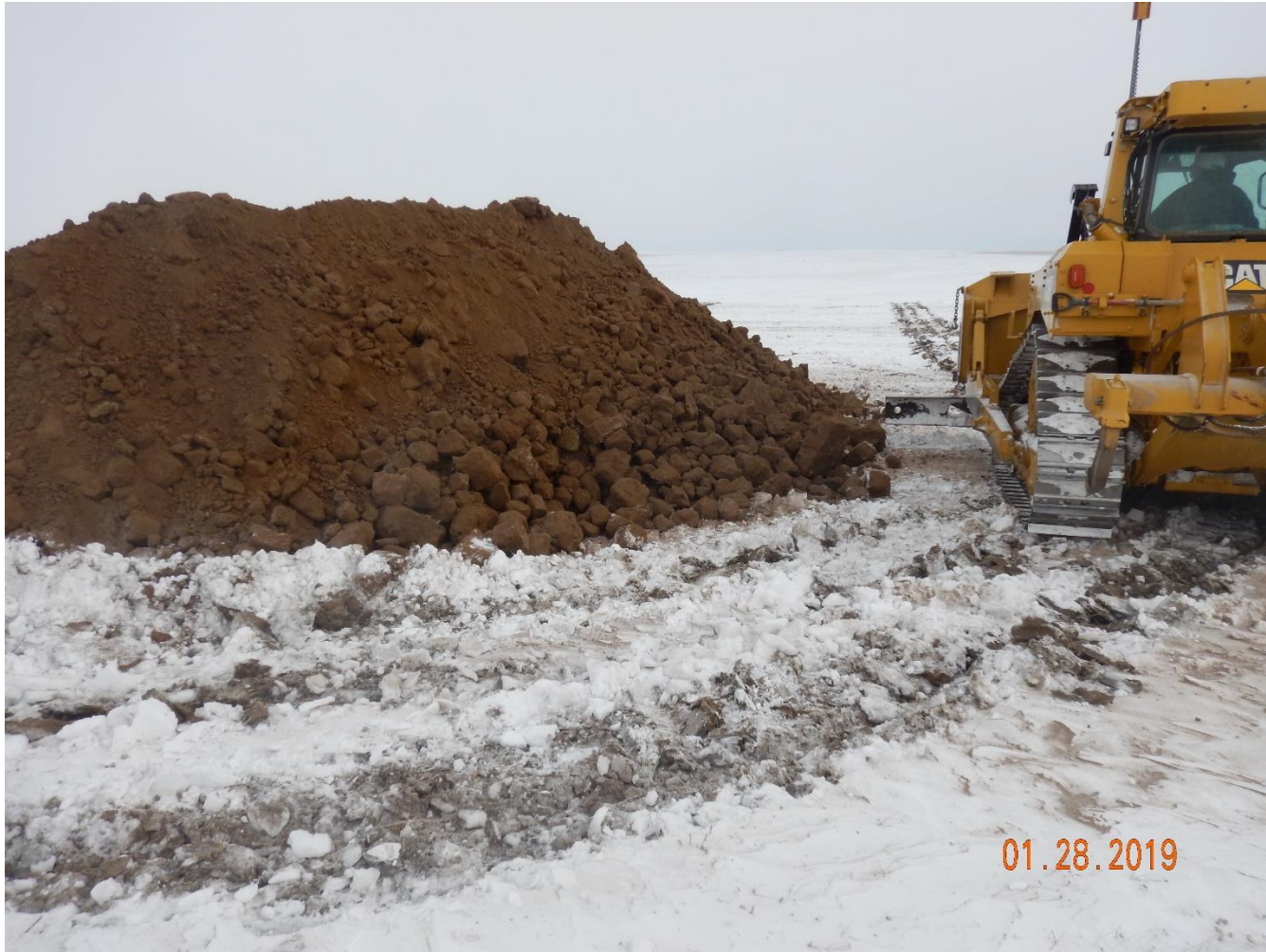
Photo 2: Photo taken from the southwest end of the location, facing east Photo shows topsoil salvage and pad construction in process. Photo also shows operator has installed surface roughening along the perimeter of the location.
