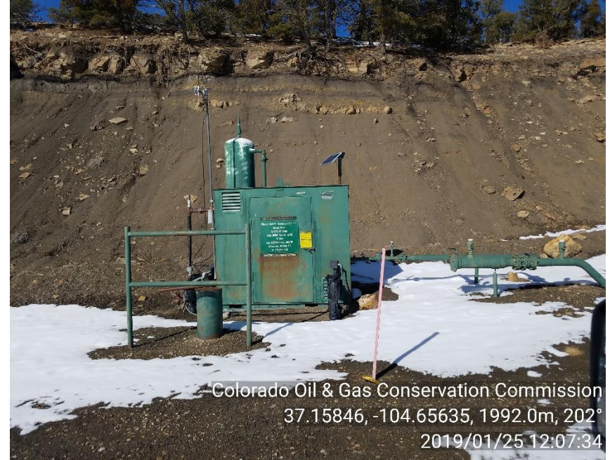
PHOTO 2: WELL SIGN/METER HOUSE
